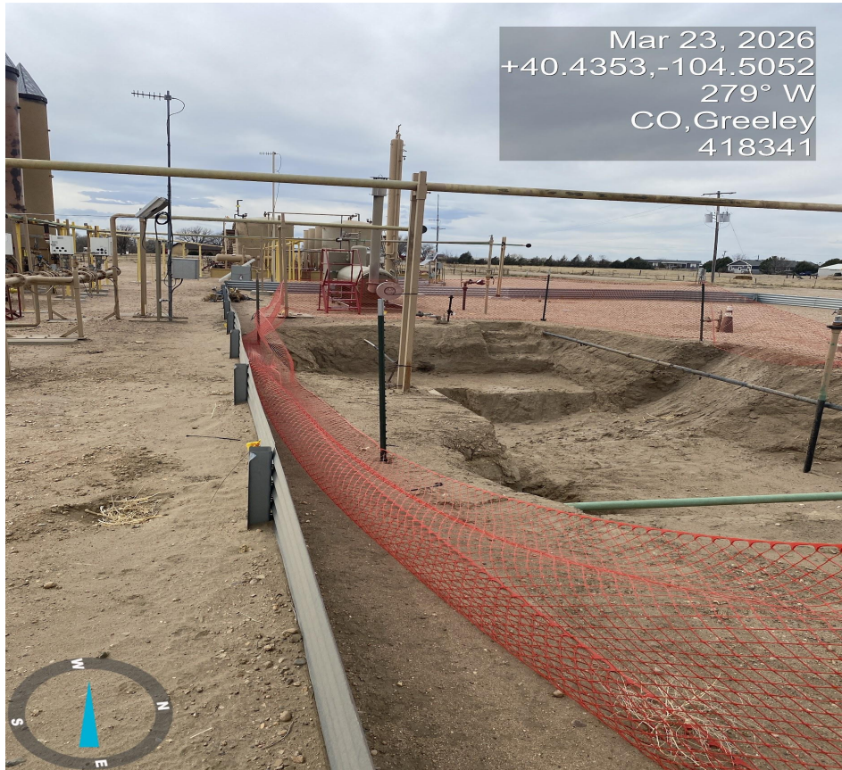
Photo 6. Photo taken from the disturbance area on the northern end showing fencing is in disrepair around excavation.
