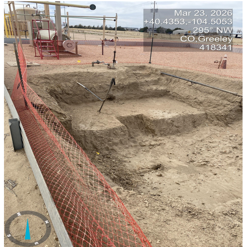
Photo 7. Photo taken from the northern end of the disturbance showing that the fencing is in disrepair.
