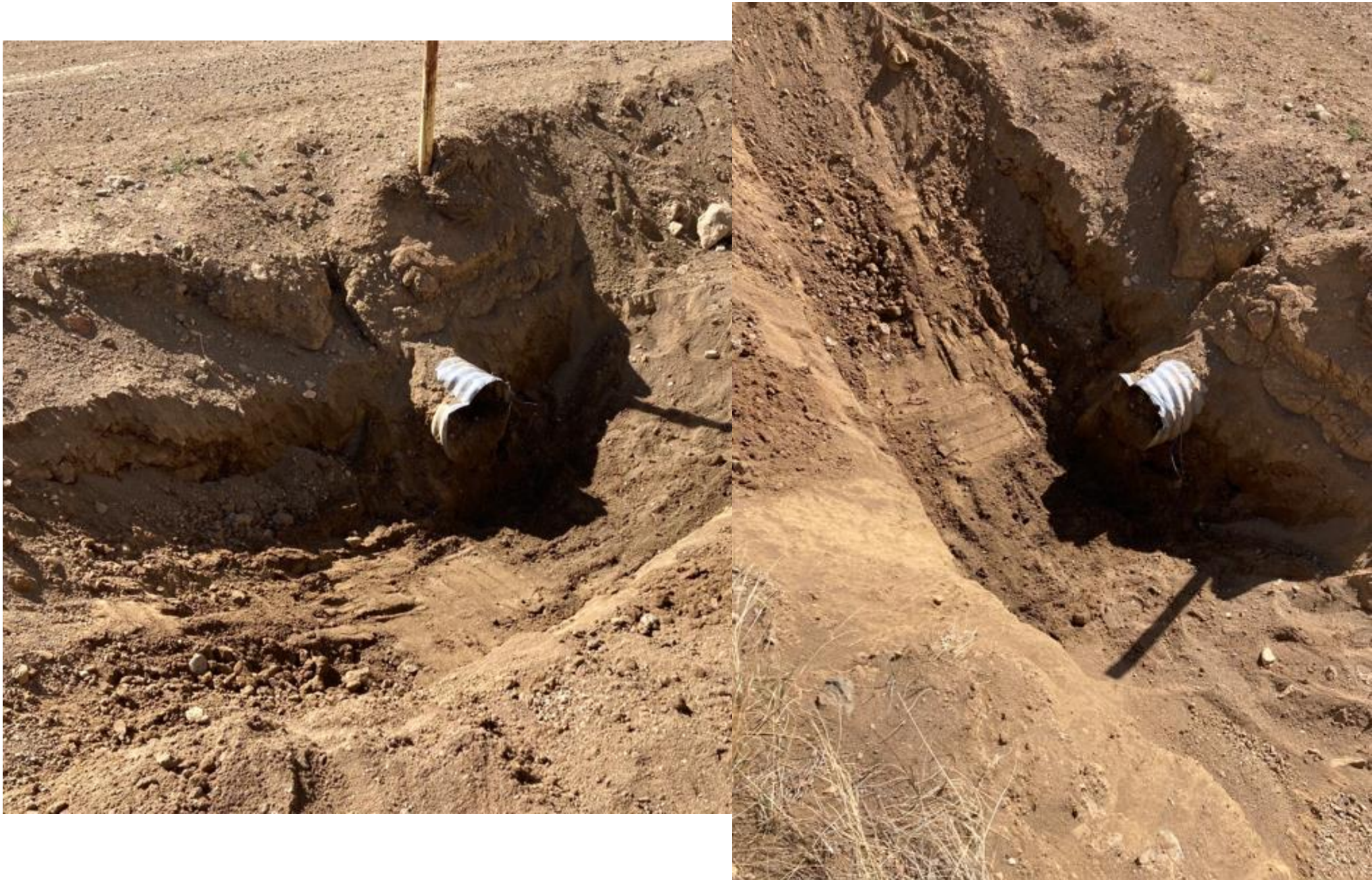
PHOTO 1: THE INLET AND OUTLET OF THE CULVERT HAS BEEN CLEANED AND RESET.
