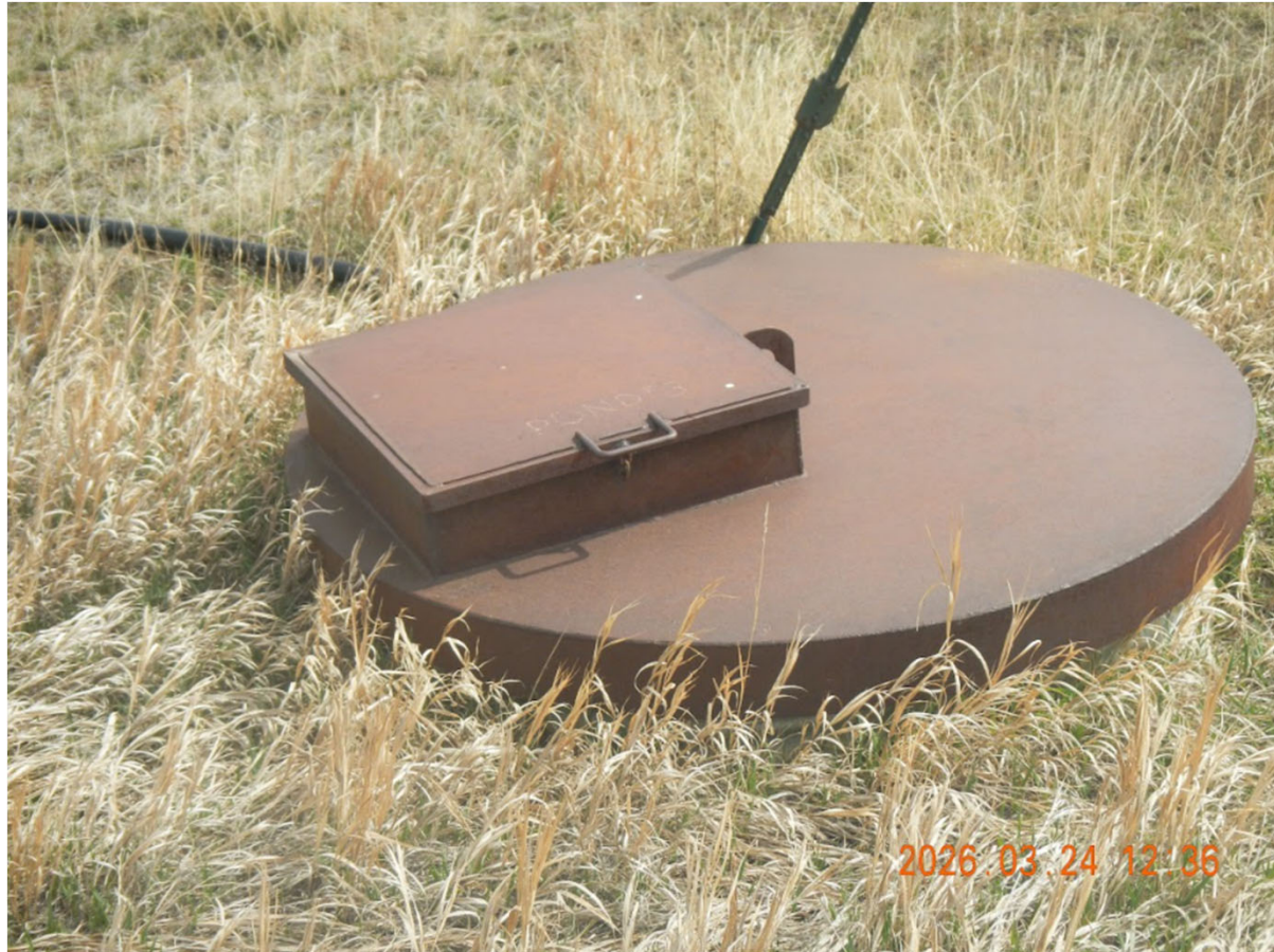
Photo 11 - Pit 3 valve can
