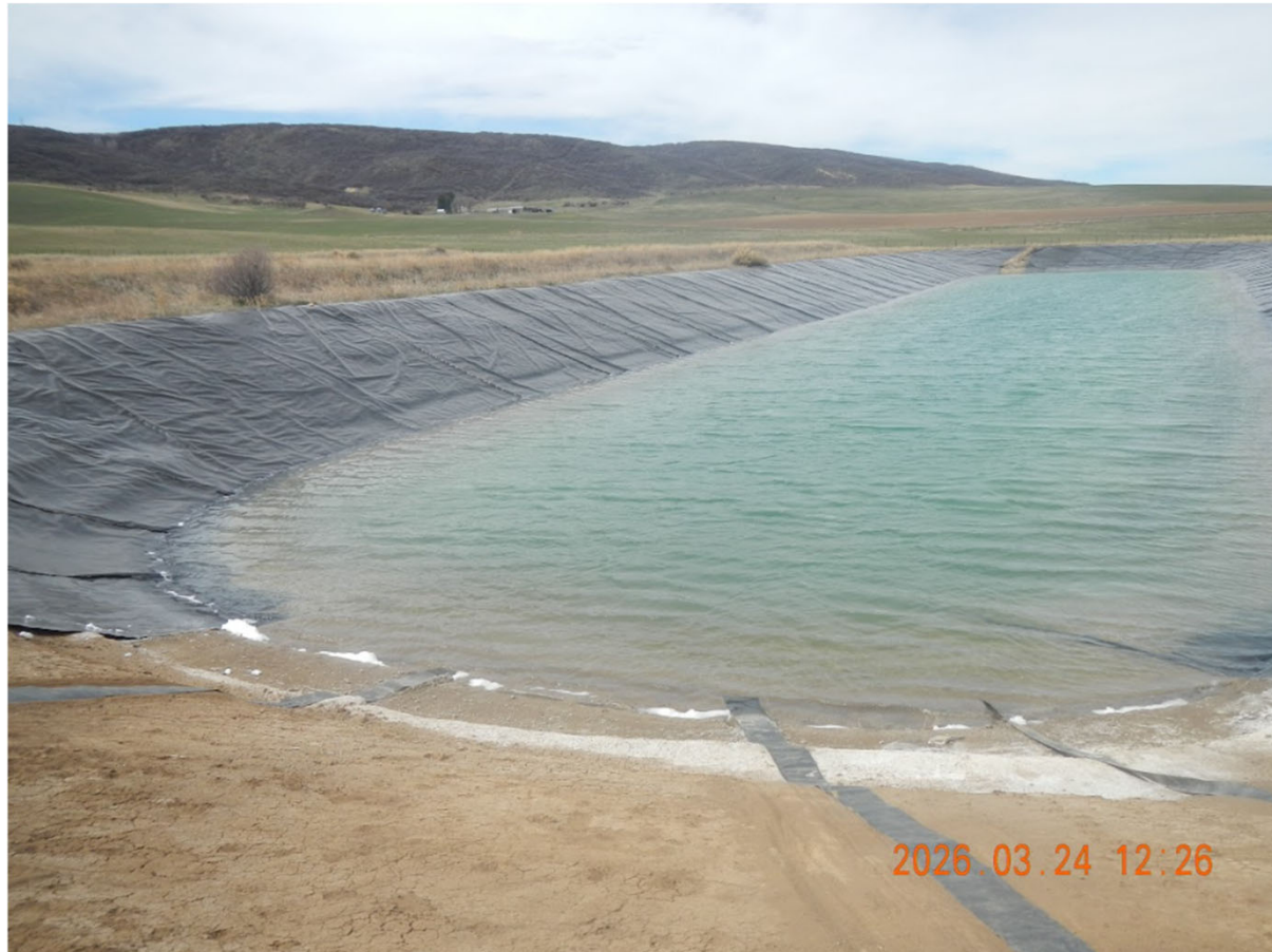
Photo 24 - Pit 7 looking West. Liner is in disrepair. Depth of fluids is approximately 12" to 24".
