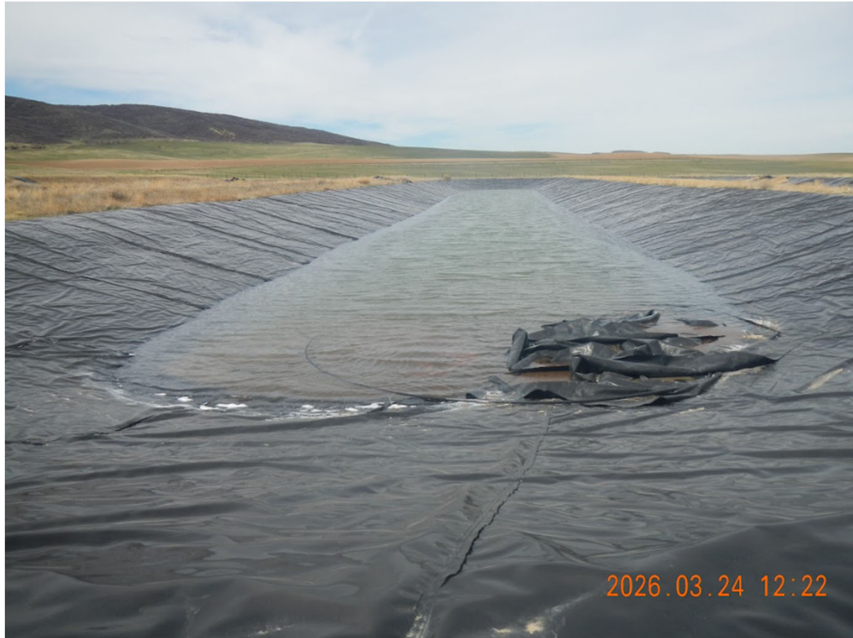
Photo 30 - Pit 9 looking West. Liner is in disrepair. Depth of fluids is approximately 12" to 24".
