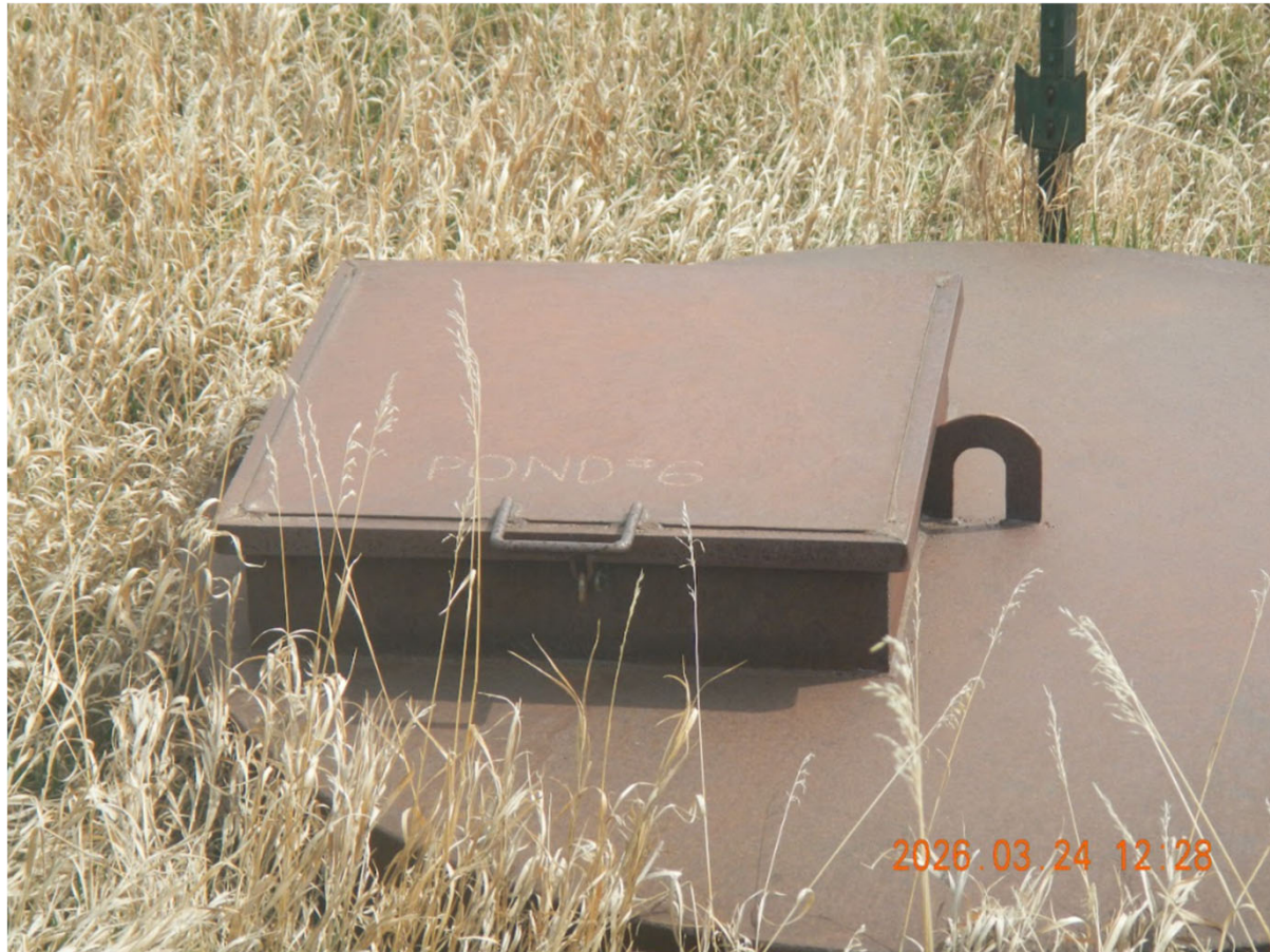
Photo 20- Pit 6 valve can
