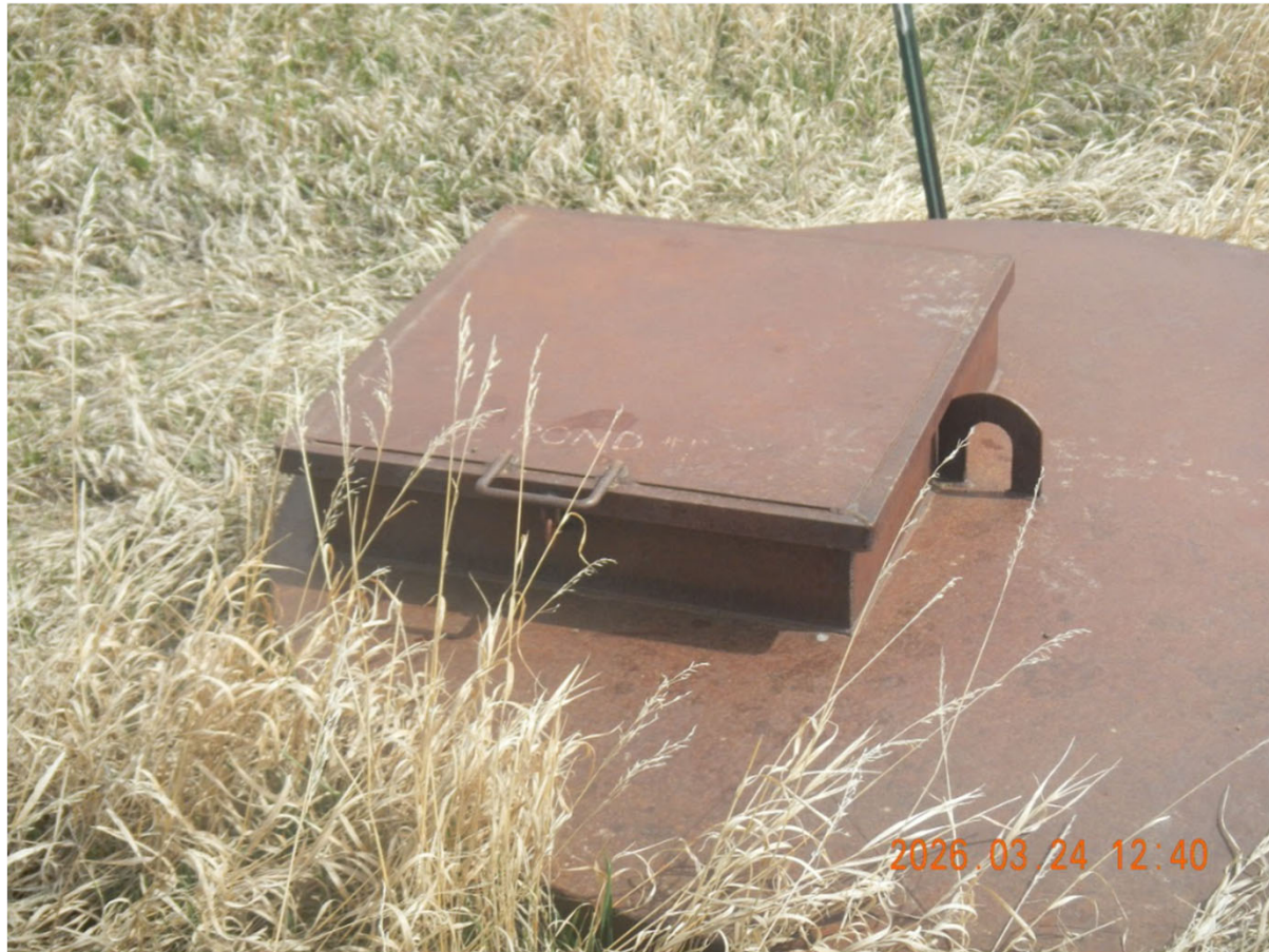
Photo 4 - Pit 1 valve can
