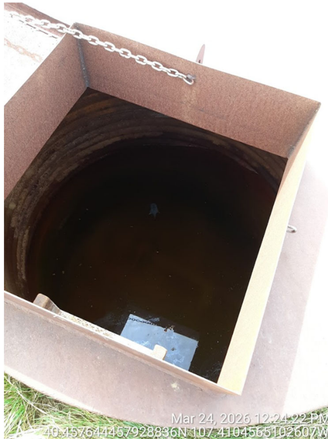
Photo 33 - Pit 10 valve can
