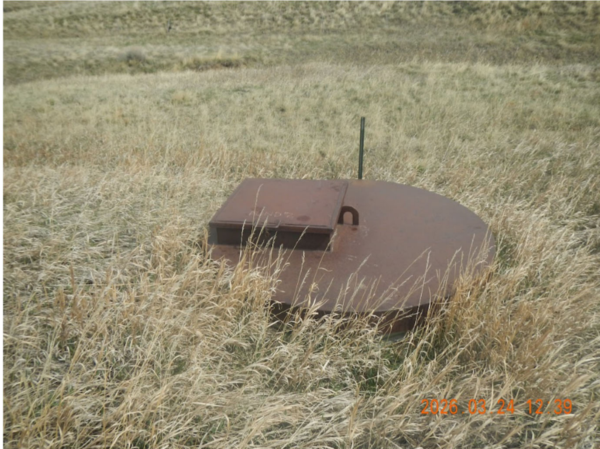
Photo 7 - Pit 2 valve can
