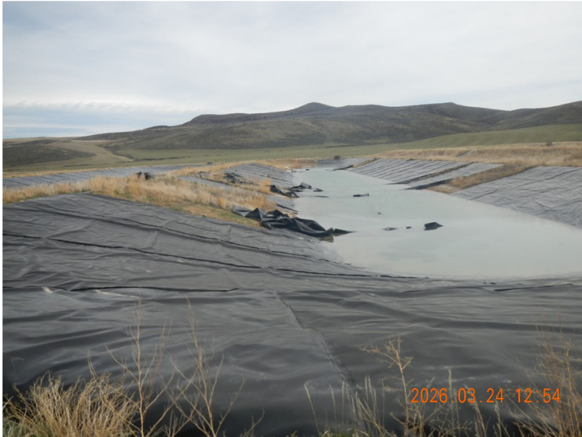
Photo 28 - Pit 8 looking East. Liner is in disrepair. Depth of fluids is approximately 12" to 24".
