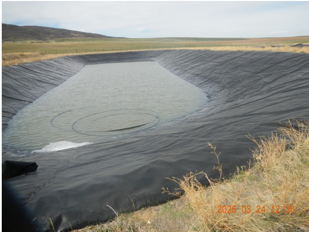
Photo 12 - Pit 3 looking west. Depth of fluids is approximately 12" to 24".
