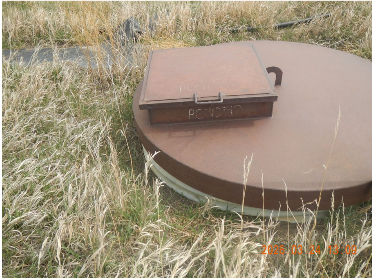
Photo 32 - Pit 10 valve can
