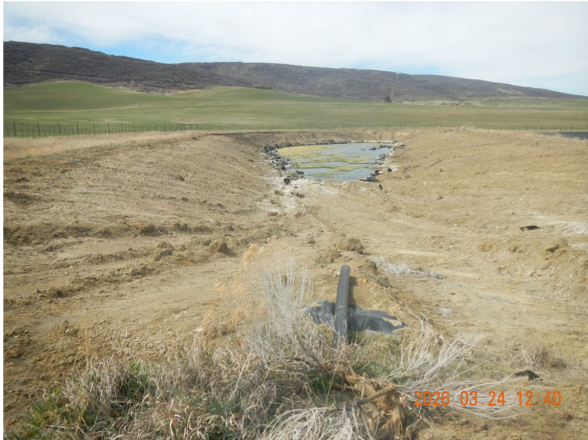
Photo 5 - Pit 1 looking west. Disturbance along the pit walls. Note that most of the liner has been removed with some liner remaining in the base of the pit.
