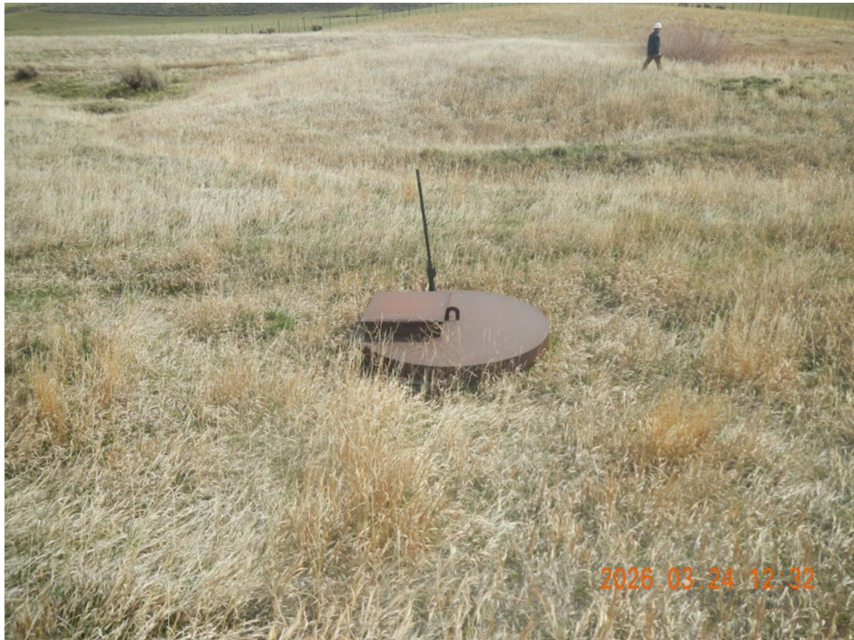
Photo 14 - Pit 4 valve can
