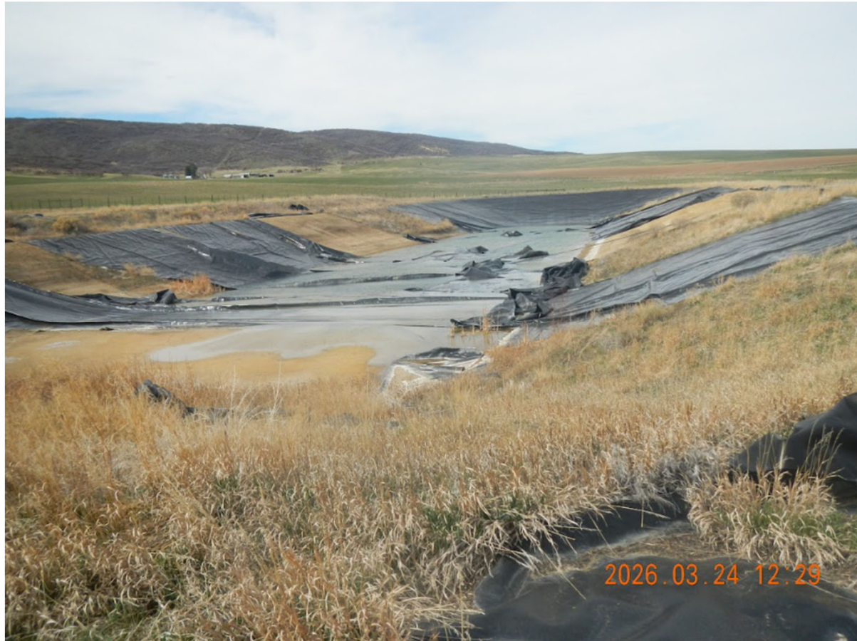
Photo 18 - Pit 5 looking west. Liner is in disrepair. Depth of fluids is approximately 12" to 24".
