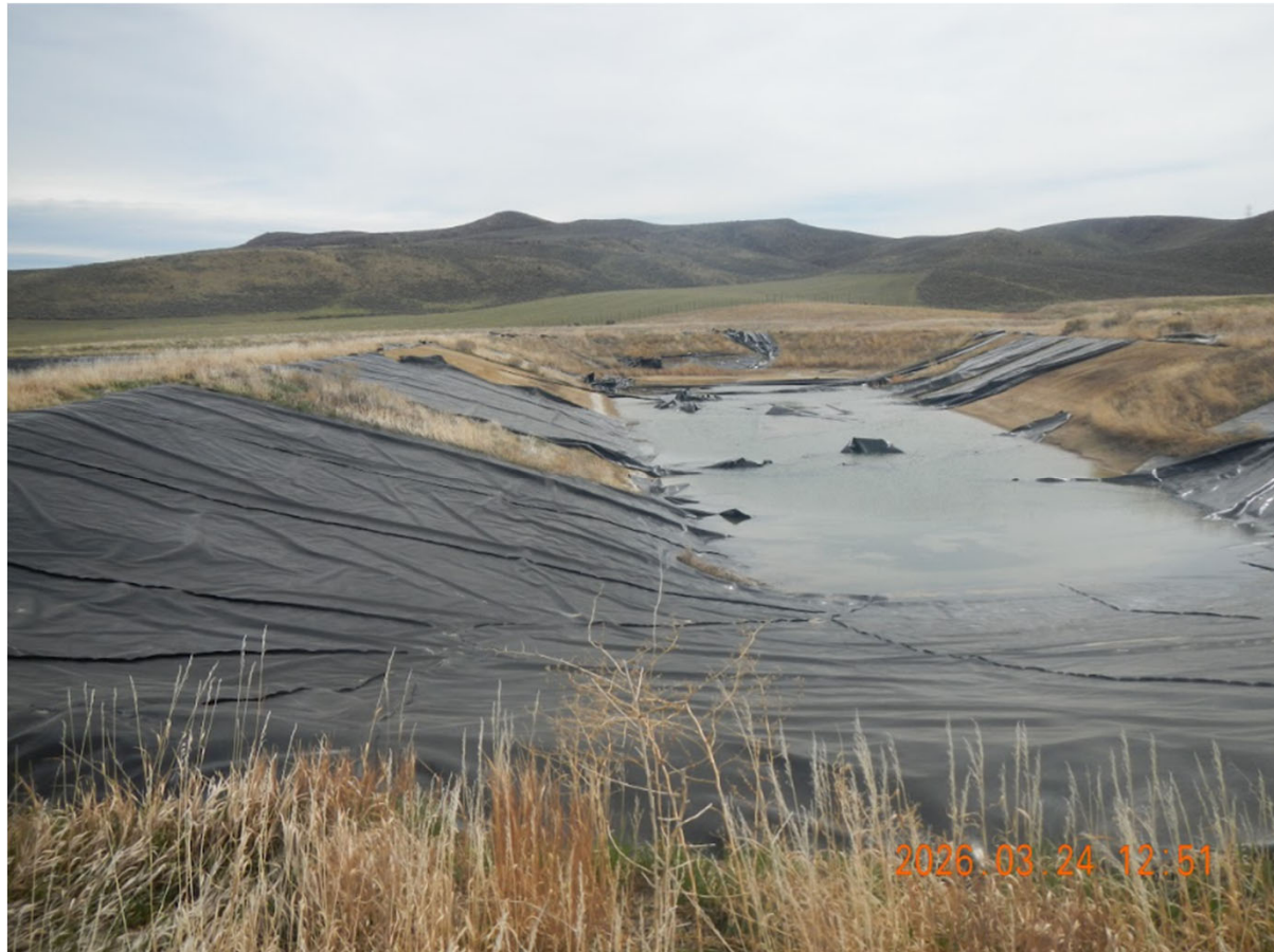
Photo 19 - Pit 5 looking east. Liner is in disrepair. Depth of fluids is approximately 12" to 24".
