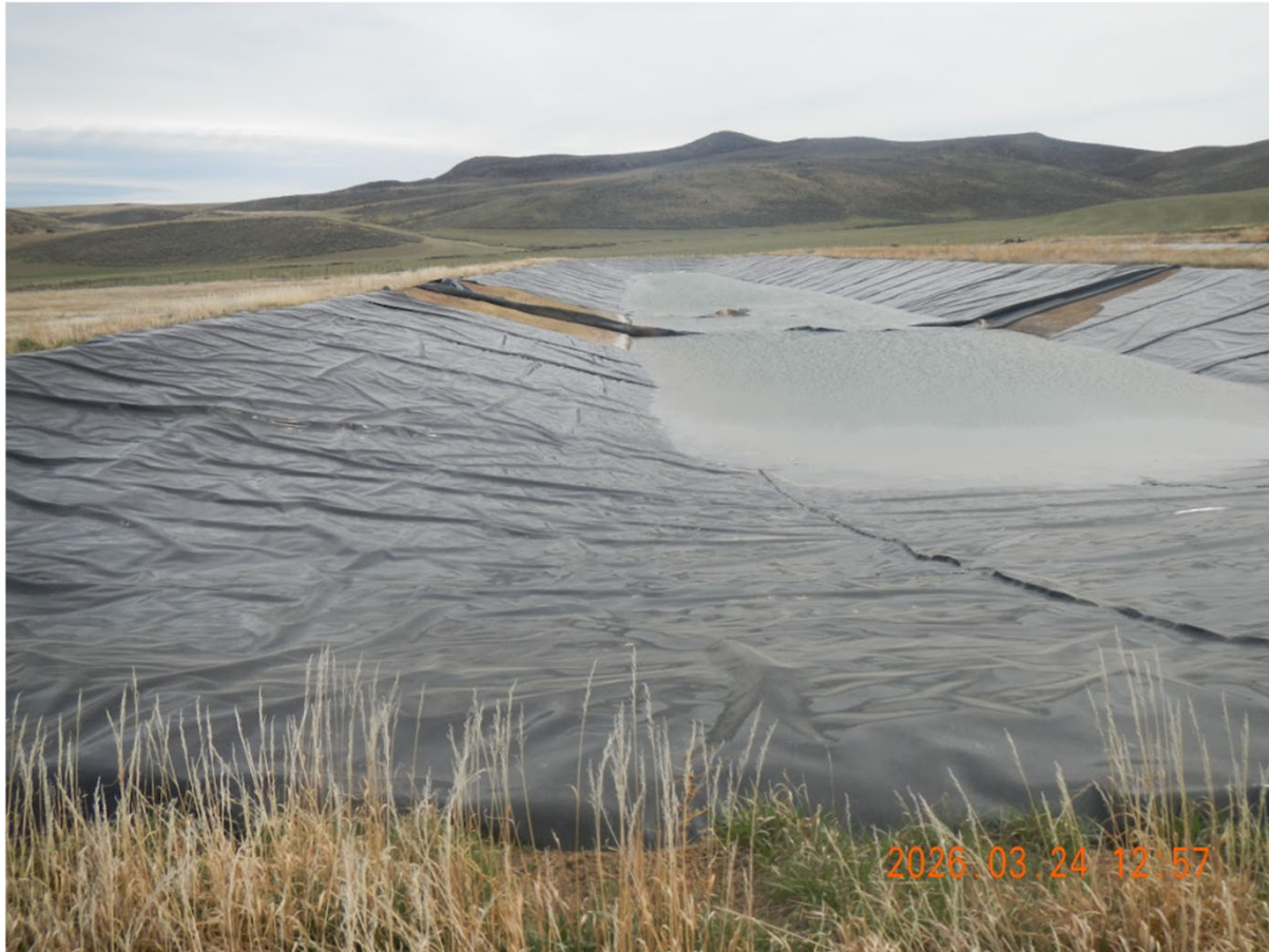
Photo 35 - Pit 10 looking East. NOTE: Liner is in disrepair. Depth of fluids is approximately 12" to 24".
