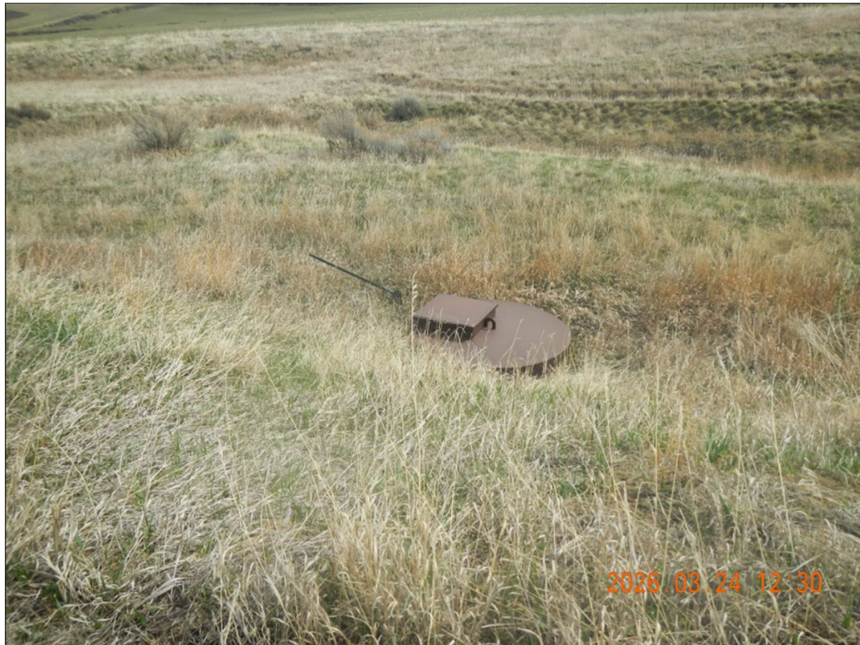
Photo 17 - Pit 5 valve can
