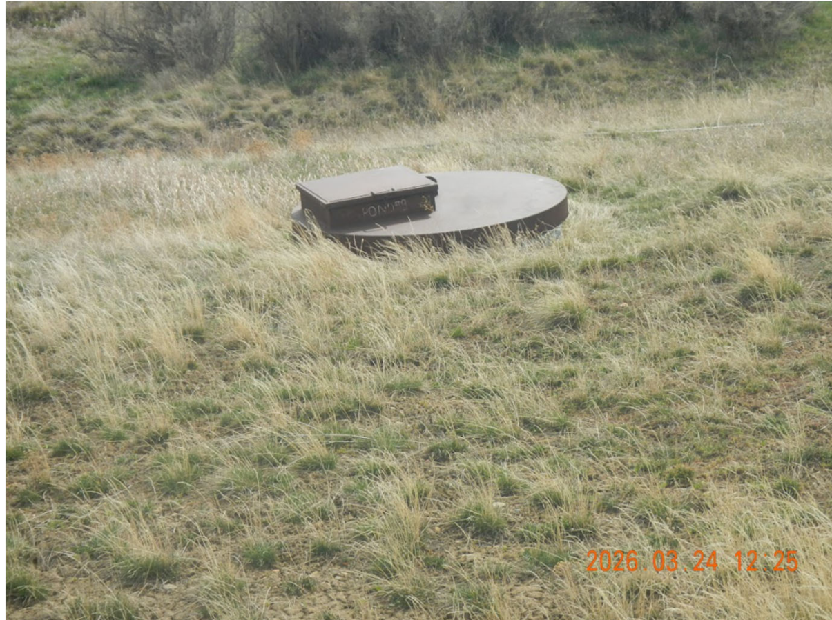
Photo 26 - Pit 8 valve can
