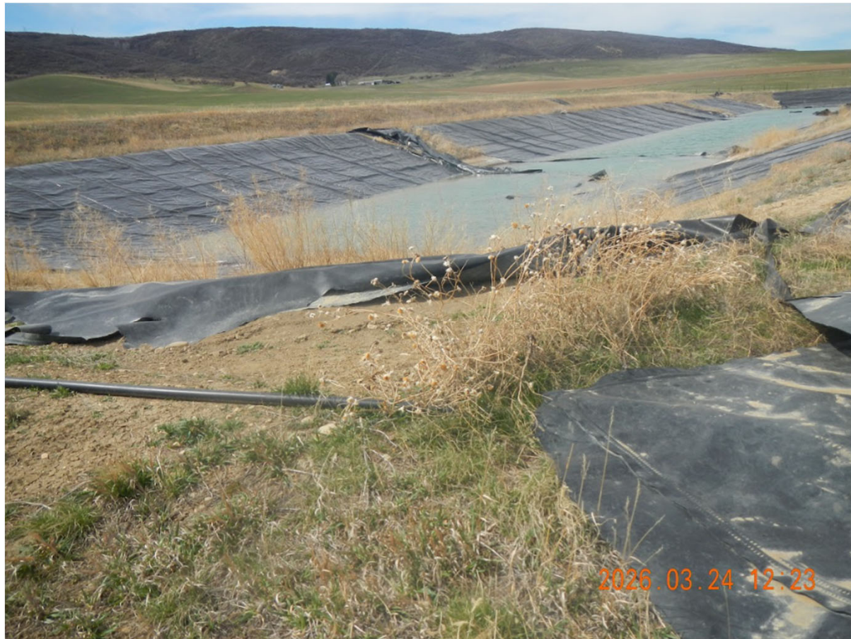
Photo 27 - Pit 8 looking West. Liner is in disrepair. Depth of fluids is approximately 12" to 24".
