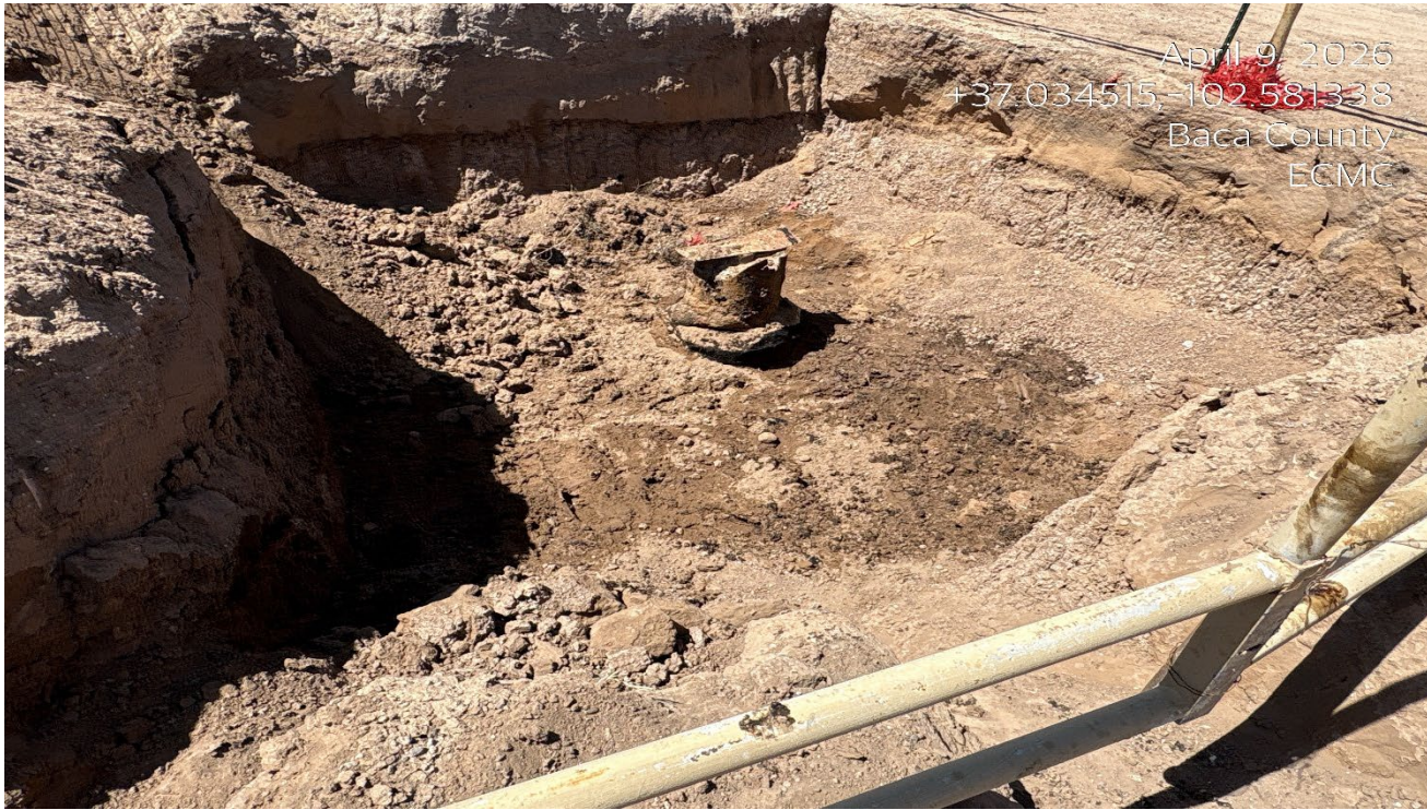
Photo 5. Facing toward the cut and capped well. There appears to be wet impacted soils around the abandoned well.
