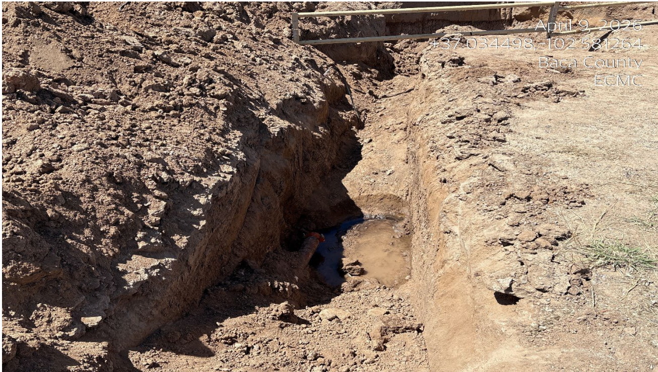
Photo 4. Near the abandoned well is a capped flowline. There is standing water at this area from a possible leak of the flowline.
