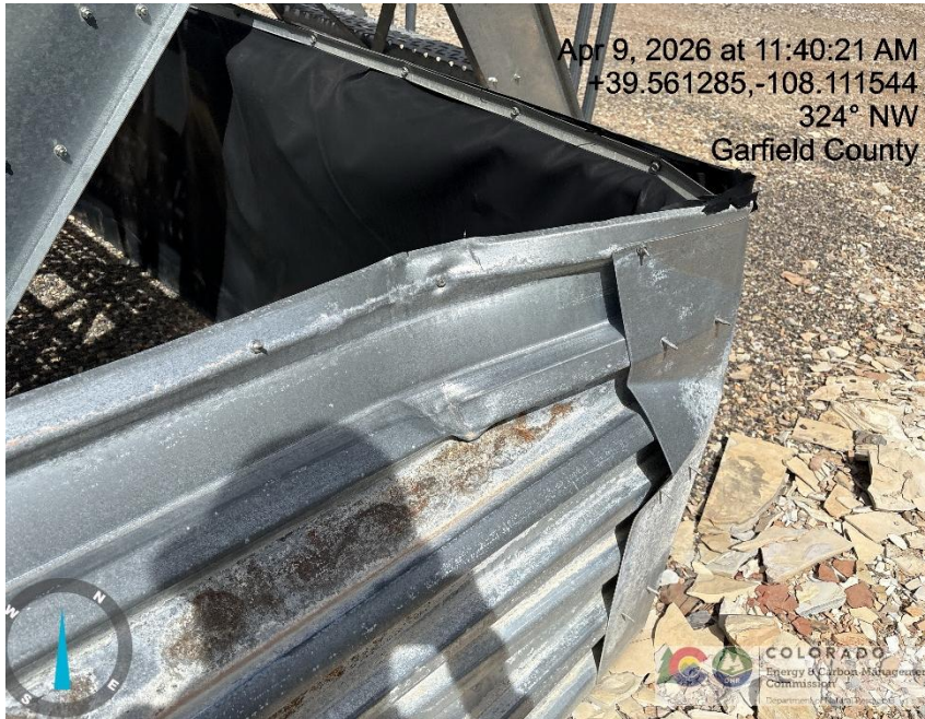
Photo # 6534 Damage to secondary containment
