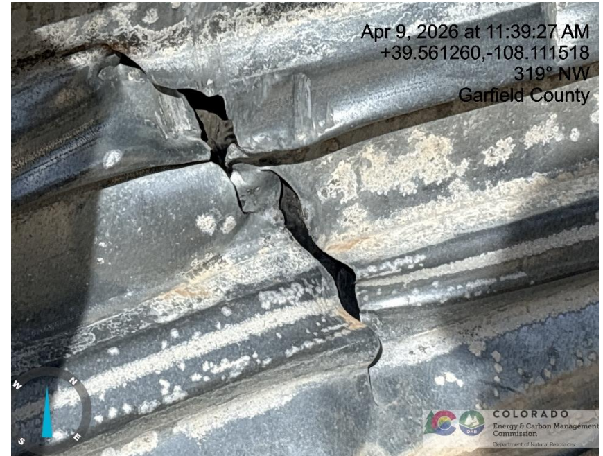
Photo # 6535 Damage to secondary containment
