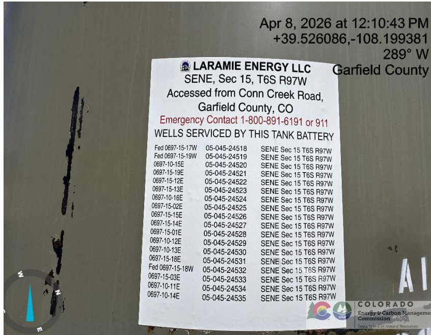
Photo # 6202 Battery sign
