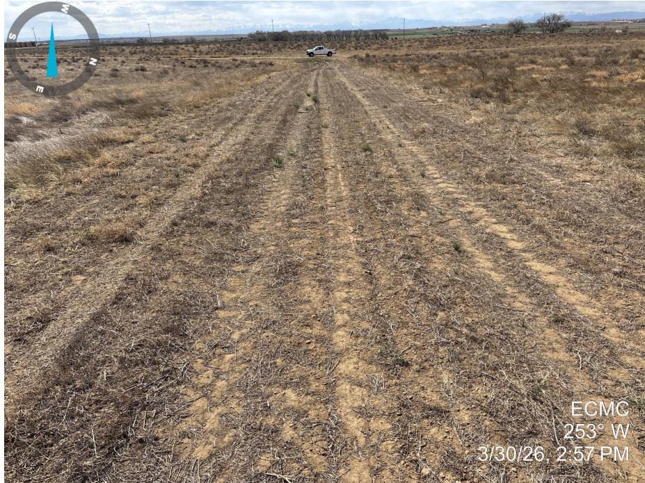
Photo 7. Photo taken of the access road to the well location, facing west. Photo illustrates that final reclamation activities appear to have taken place along the road, but vegetation has not established to Rule 1004 standards.
