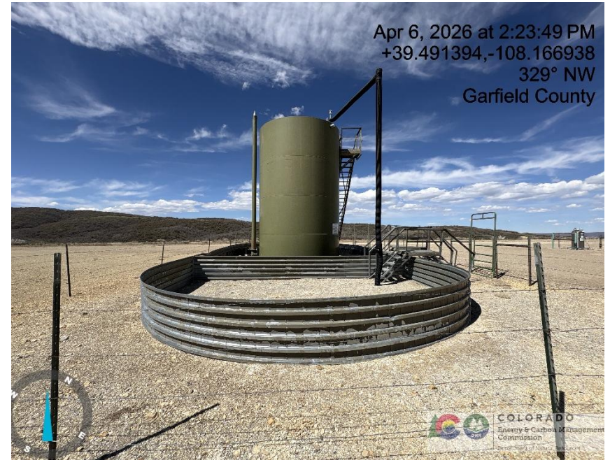
Photo # 5455 Tank battery lacks required signage
