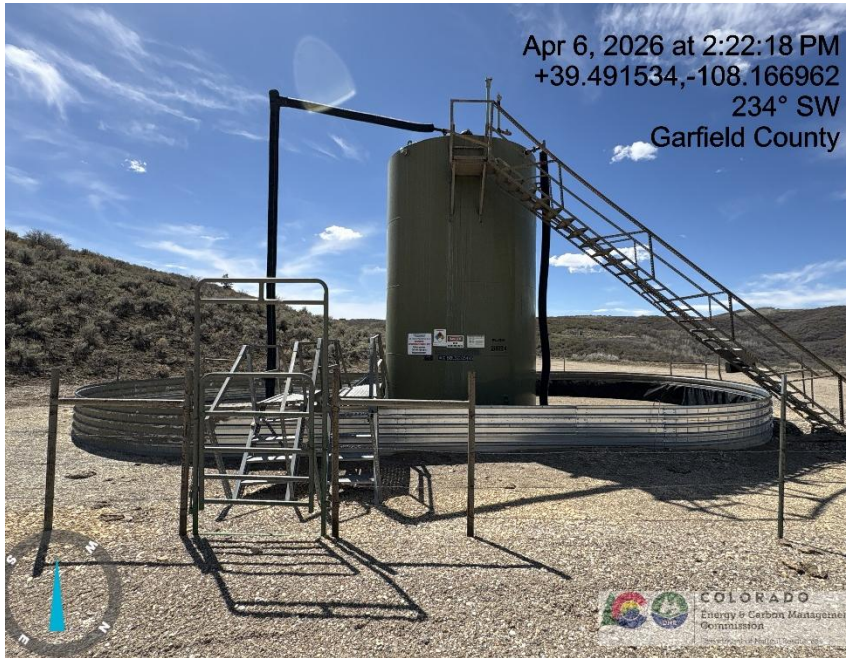
Photo # 5452 Tank battery lacks required signage
