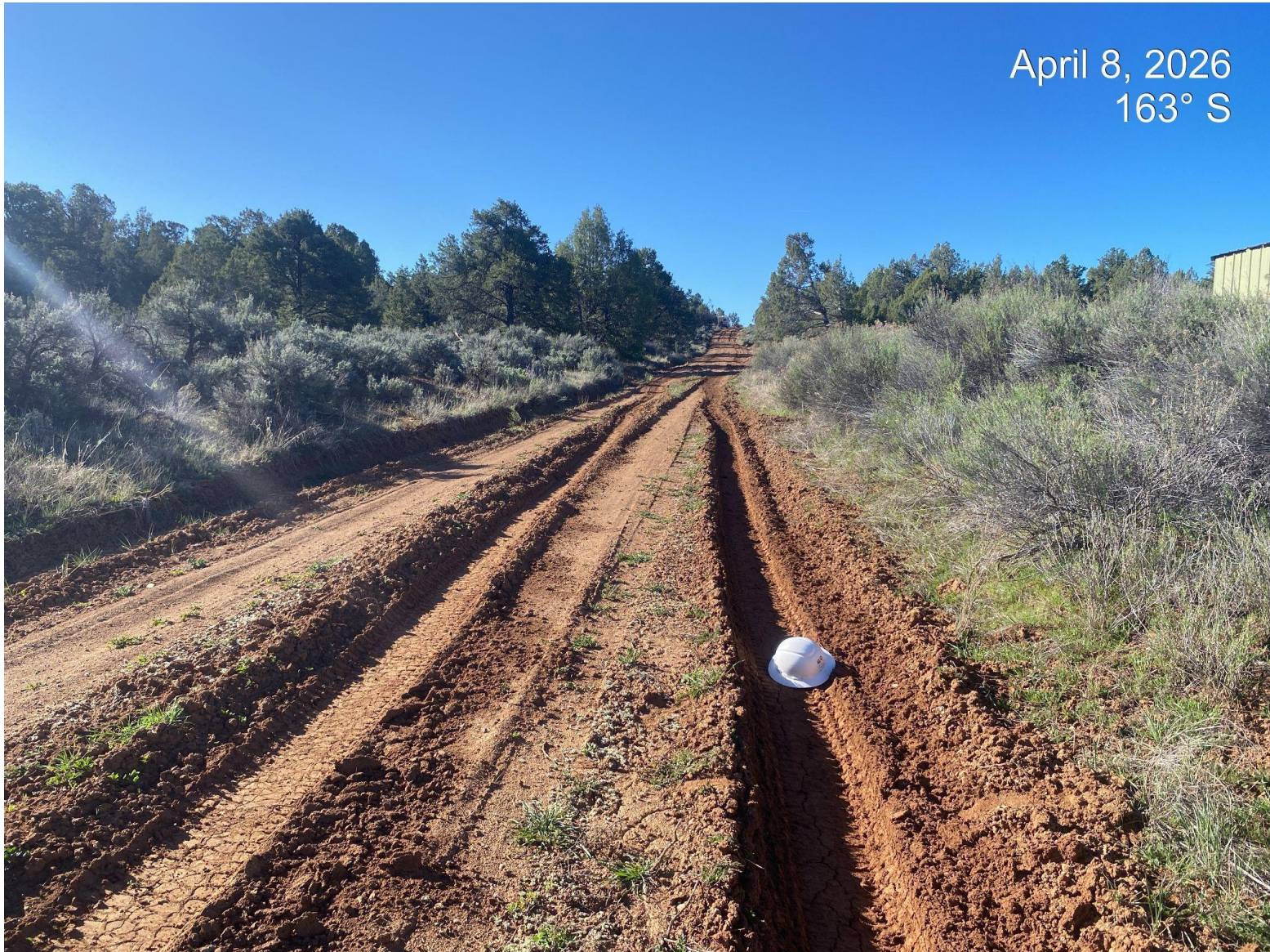
Photo 3. Deep rutting along the access road.
