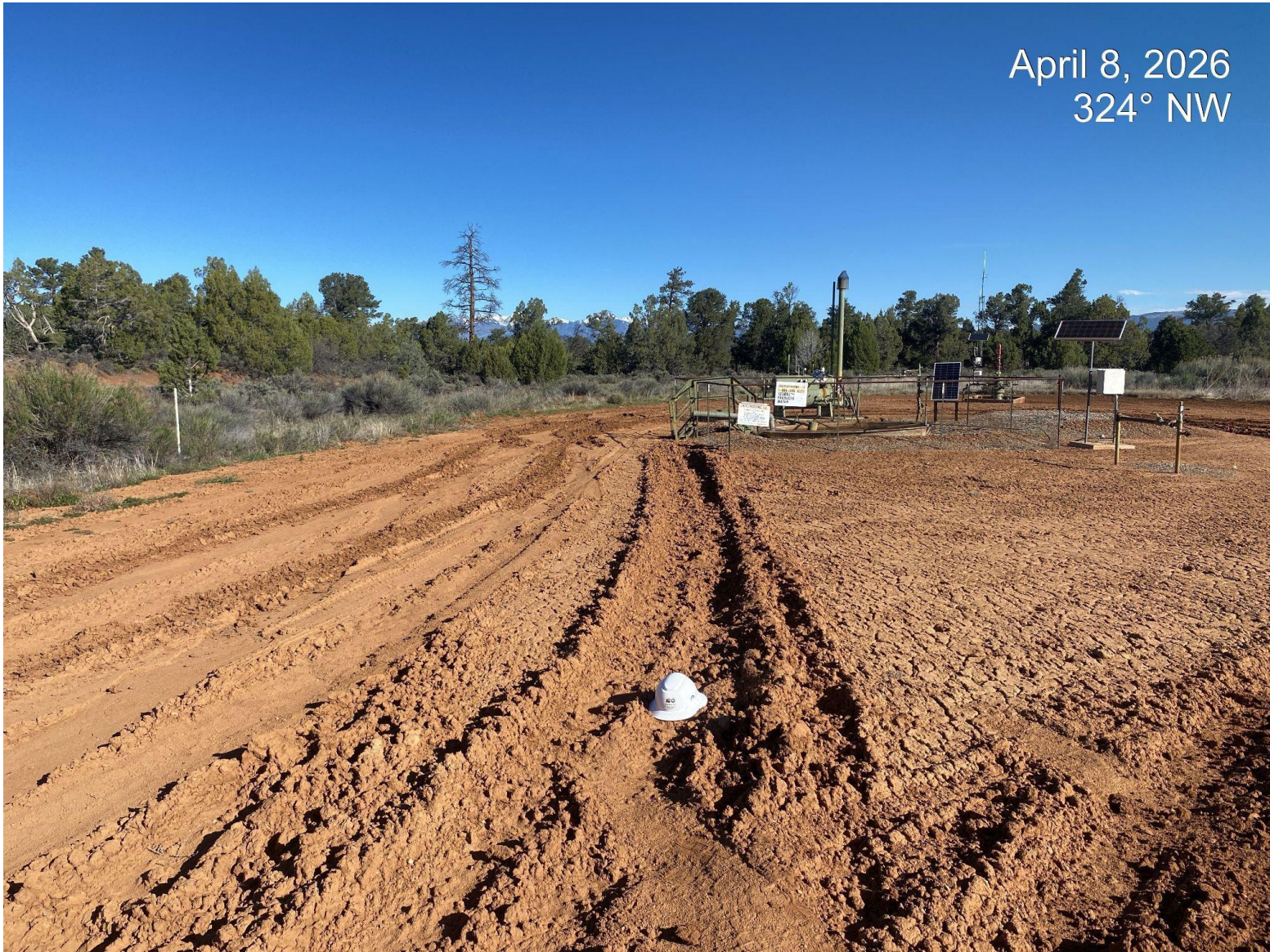
Photo 2. View of deep rutting occurring on the active pad.
