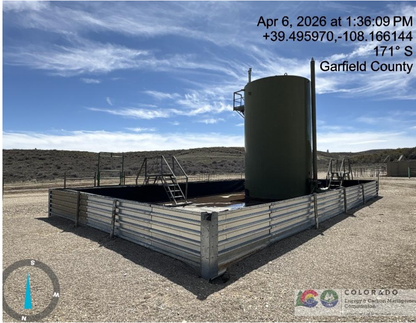
Photo # 5236 Tank battery lacks required signage
