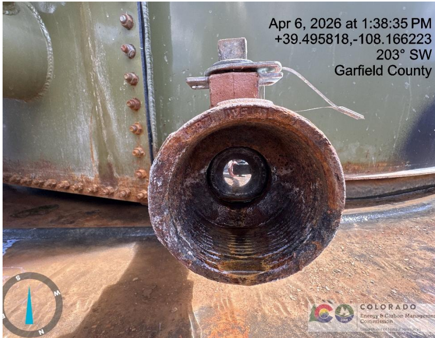
Photo # 5238 Open ended load line
