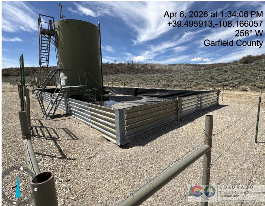
Photo # 5234 Tank battery lacks required signage
