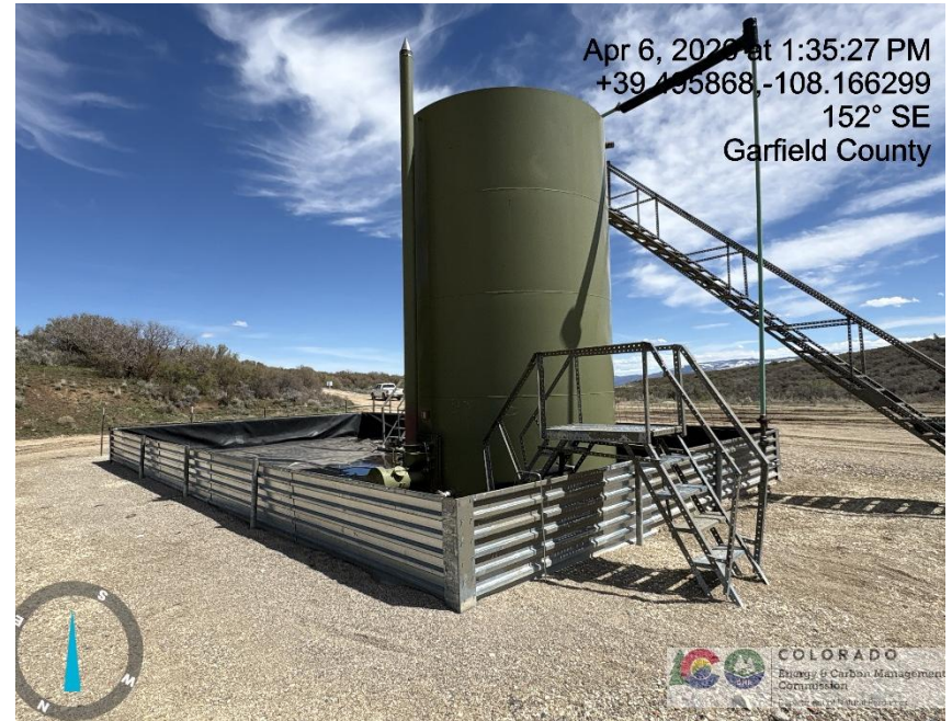
Photo # 5235 Tank battery lacks required signage
