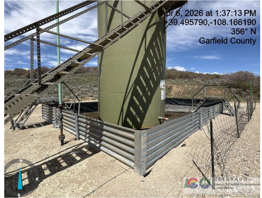
Photo # 5237 Tank battery lacks required signage
