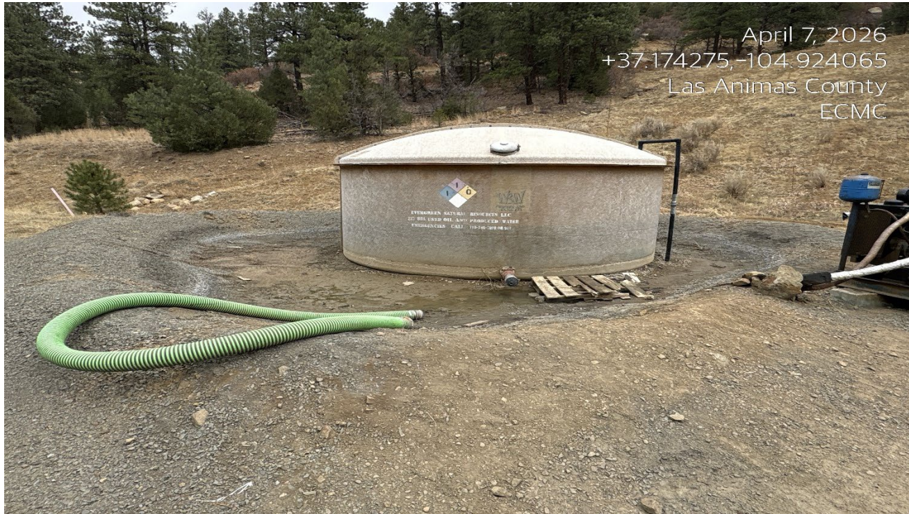
Photo 3. There was wet soils and a dripping leak at the tank which was inside secondary containment.
