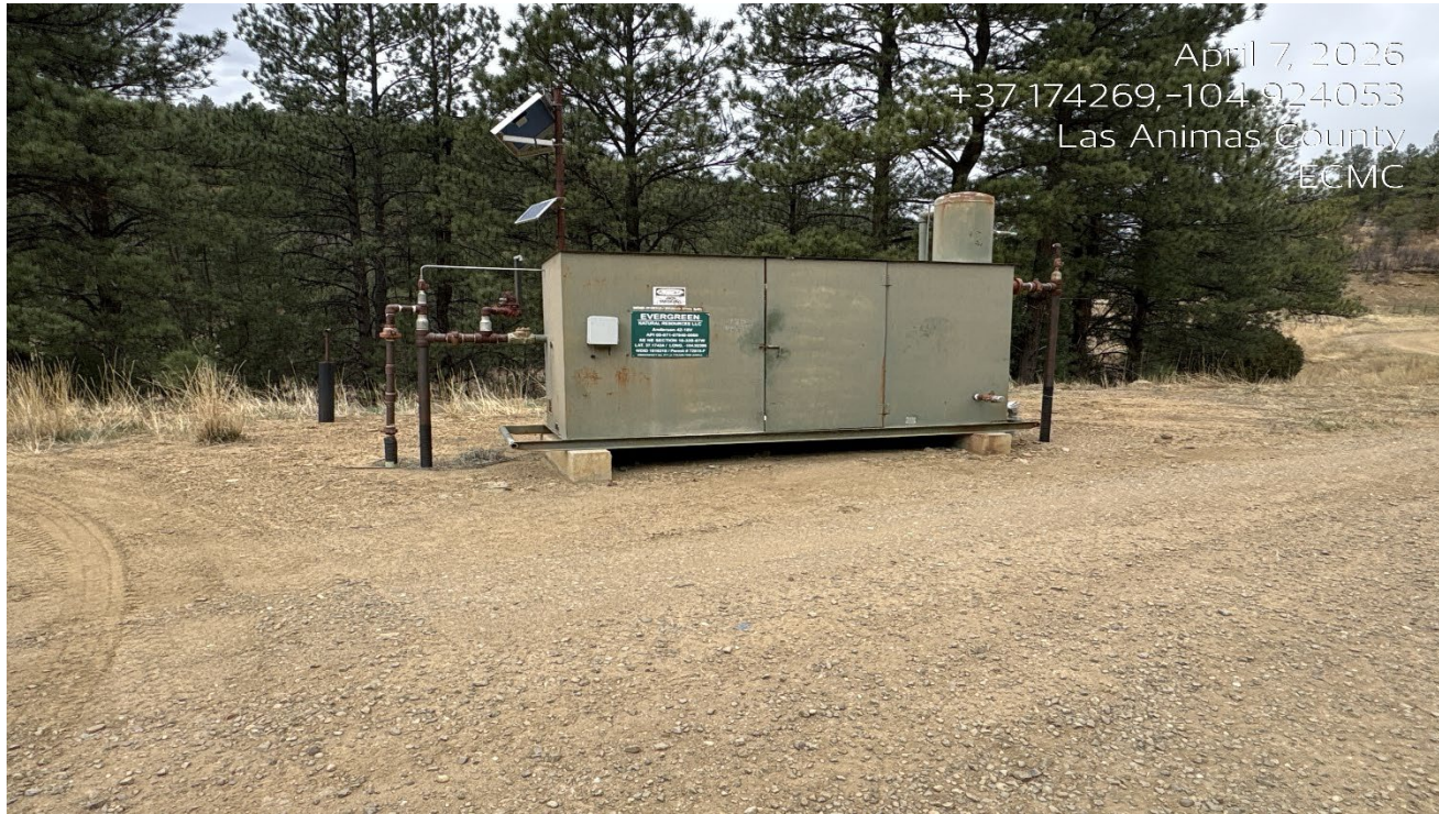
Photo 1. Well sign posted at meter shed.
