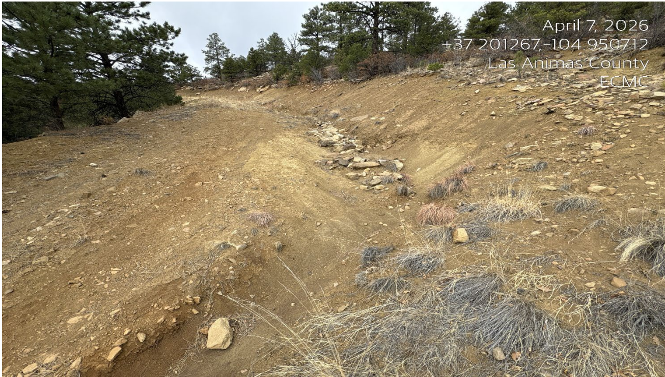
Photo 2. Facing west climbing up the road. This area has eroded and needs to be repaired and stabilized.
