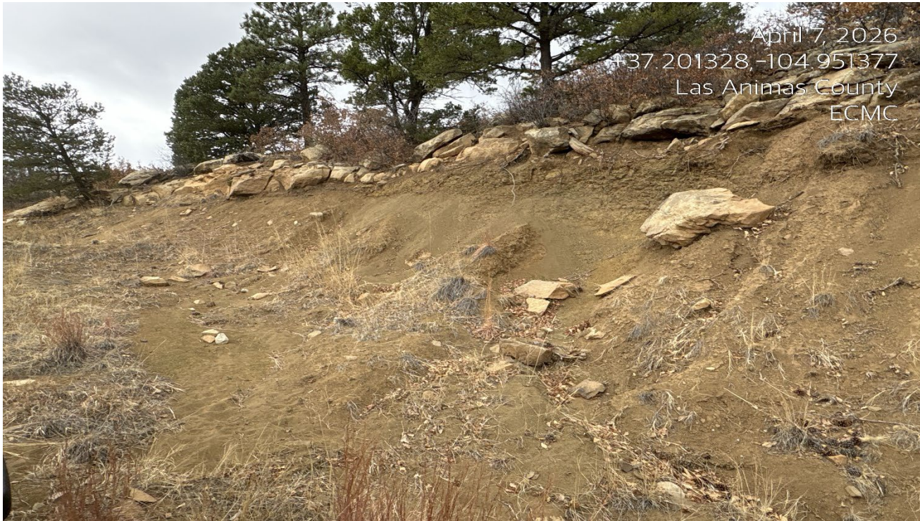
Photo 5. There is stormwater runoff causing erosion at this point which is directed down the road.
