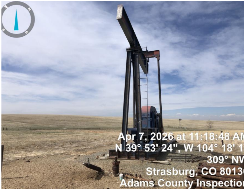
PHOTO#3 PUMPJACK/WELLHEAD T&AD
