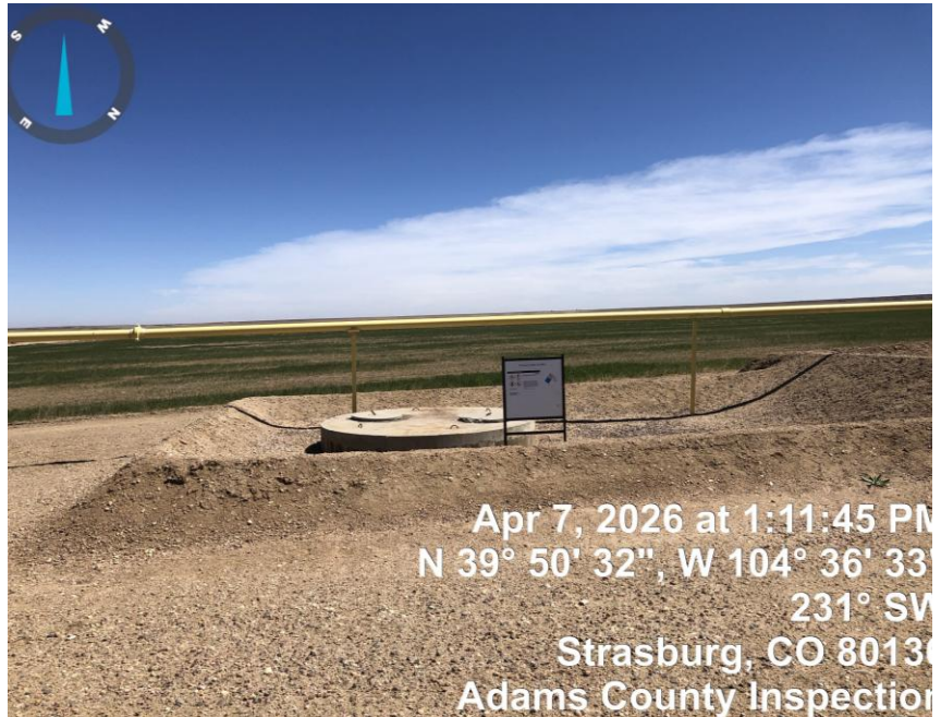
PHOTO#2 PRODUCED WATER TANK
