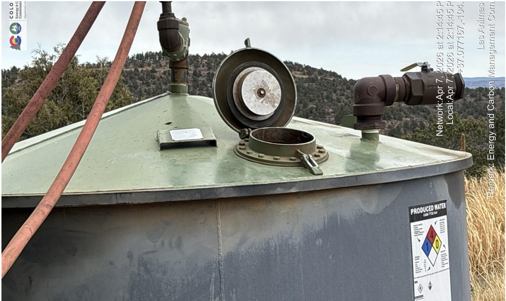
PHOTO 5: GAUGE HATCH IS STILL OPEN. THIS HATCH MUST BE KEPT CLOSED WHEN NOT GAUGING TANK.
