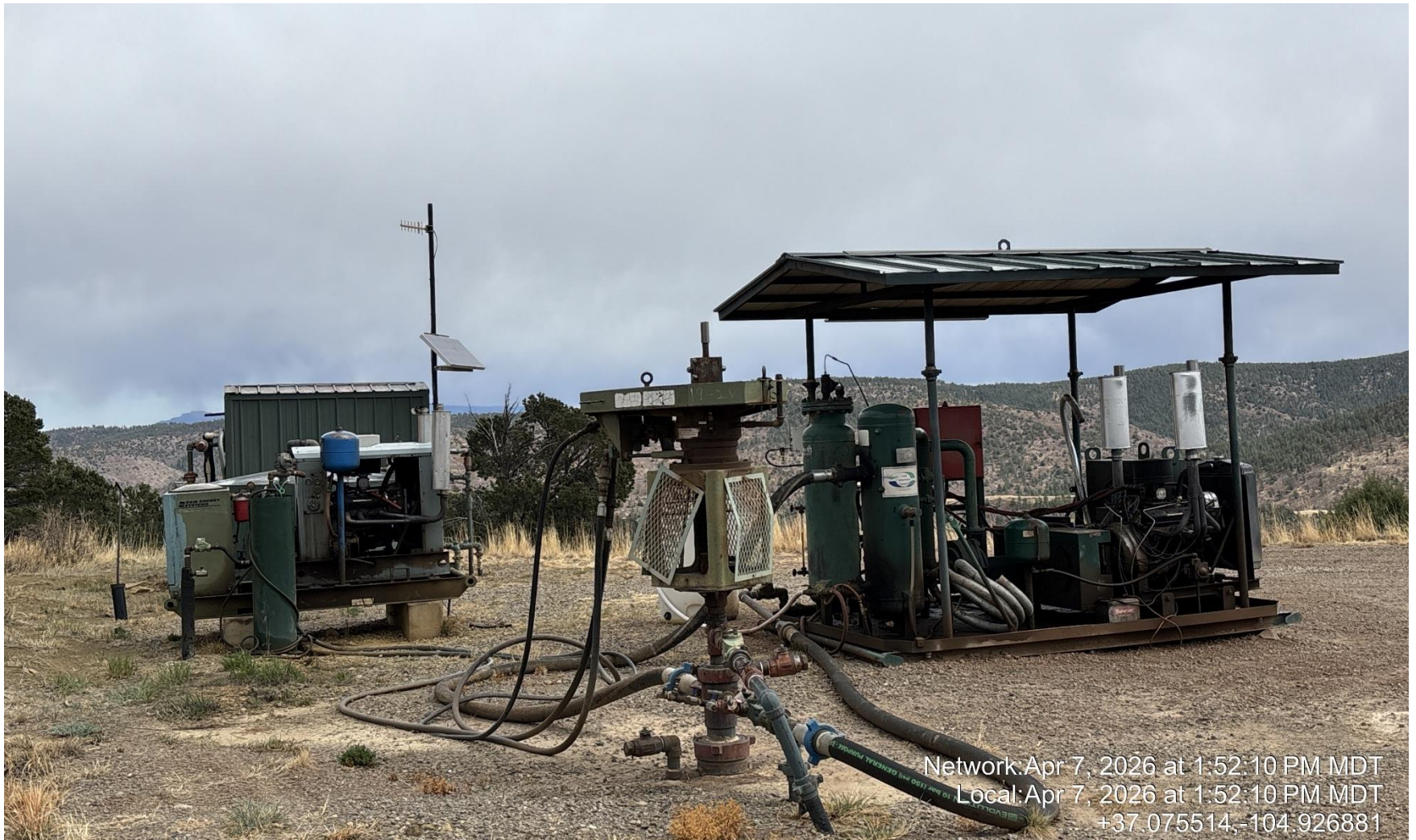
PHOTO 4: WELLHEAD AND EQUIPMENT. Vacuum pump observed on well without ECMC approval. Provide ECMC with documentation showing approval of use of vacuum pump PER RULE 432. CA DATE 4/23/2026.
