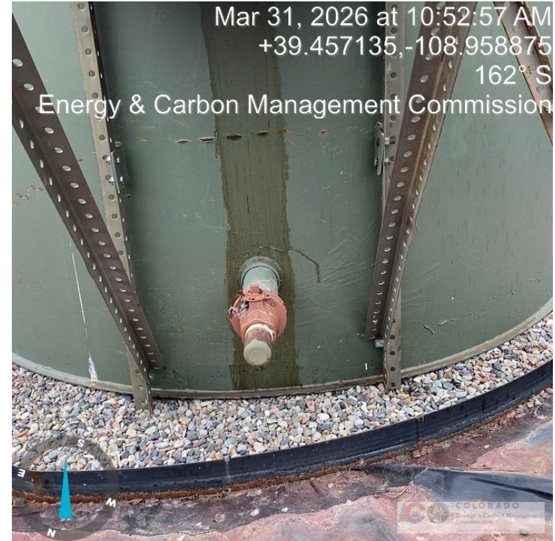
Stain on side of condensate tank.
