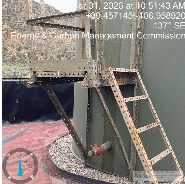
Stain on side of condensate tank.
