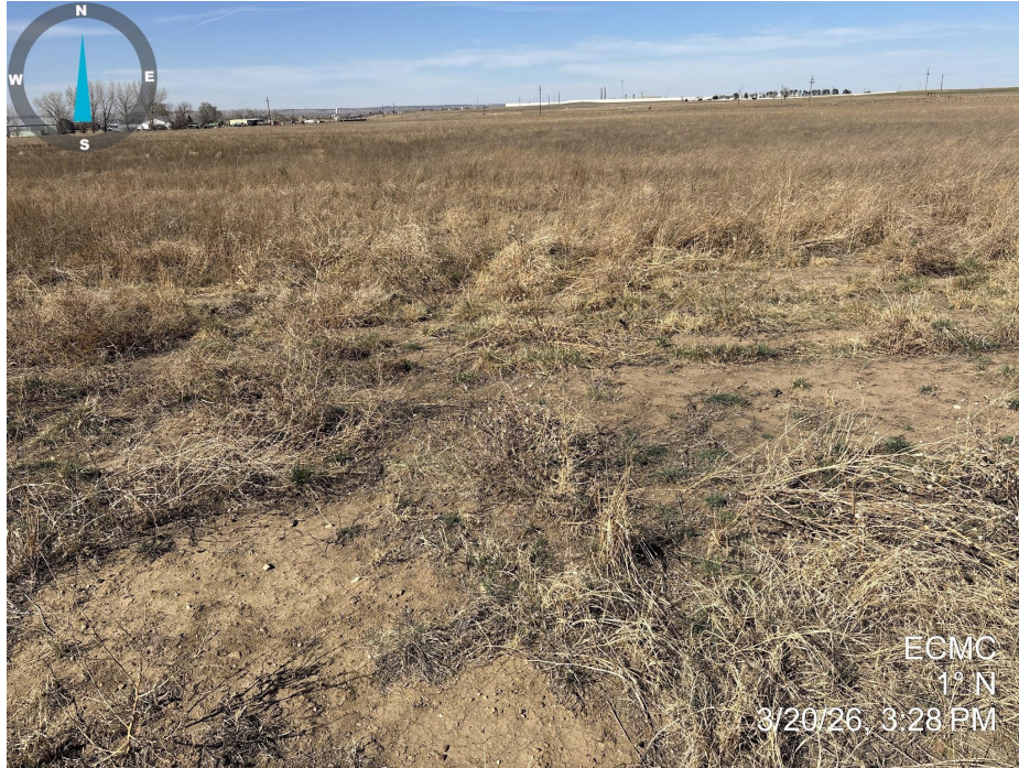
Photo 1. Photo taken of the well location, facing north. Photo illustrates that final reclamation activities appear to have taken place at the location, but vegetation establishment does not yet meet Rule 1004 standards.
