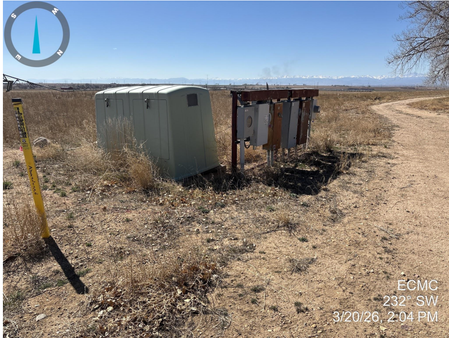
Photo 9. Photo taken of the tank battery location, facing southwest.
