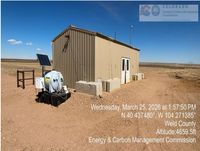
Photo 3 – Gas Lift Injection Meters
