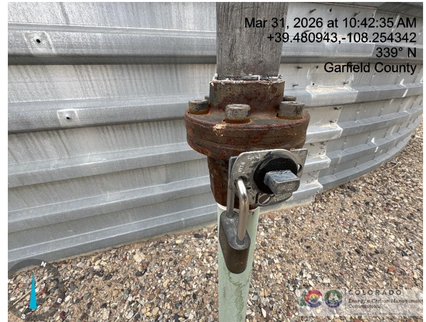
Photo # 3970 Unused flowline locked out but lacks tag/not in compliance with CECMC Rules
