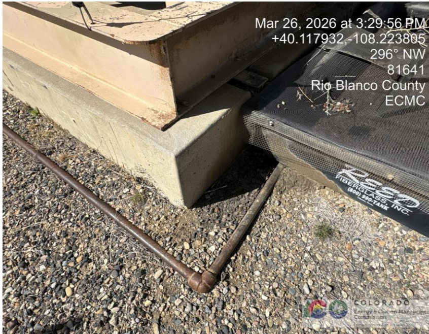
Photo # 3953 Stained soil
