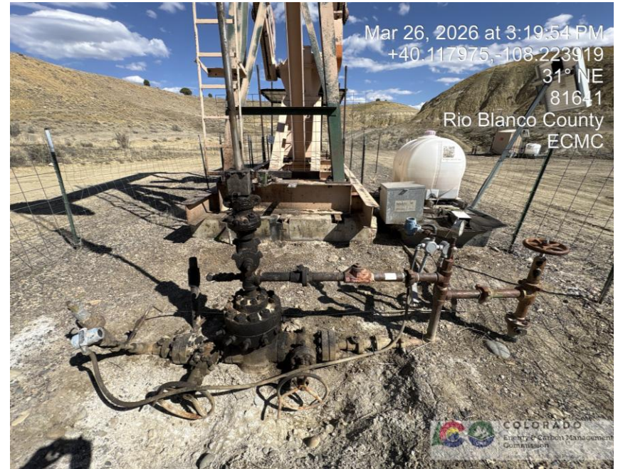
Photo # 3943 Oily waste and stained soil
