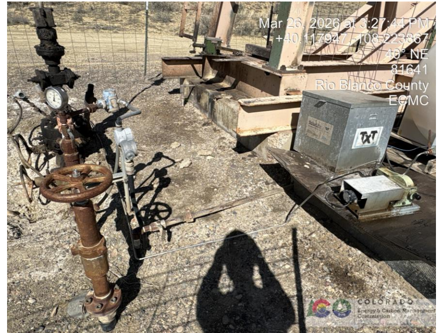
Photo # 3951 Oily waste and stained soil
