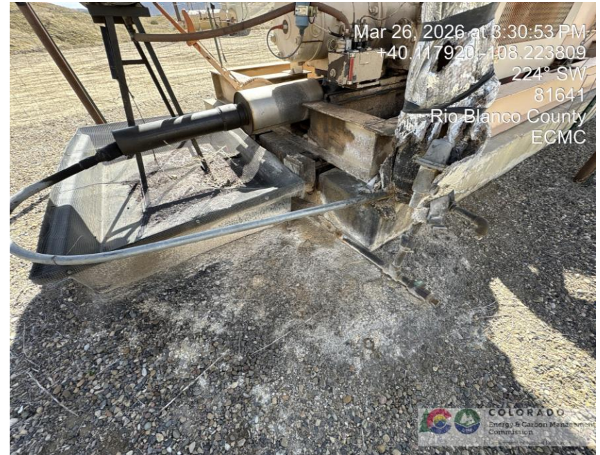
Photo # 3954 Stained soil
