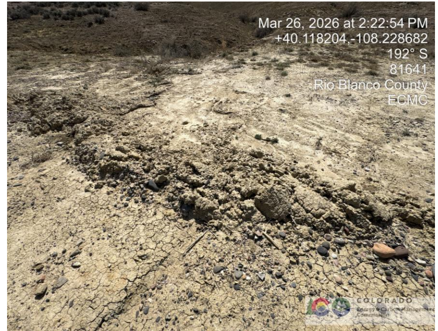
Photo # 3919 Failure to minimize erosion & transport of sediment off location/insufficient BMP's
