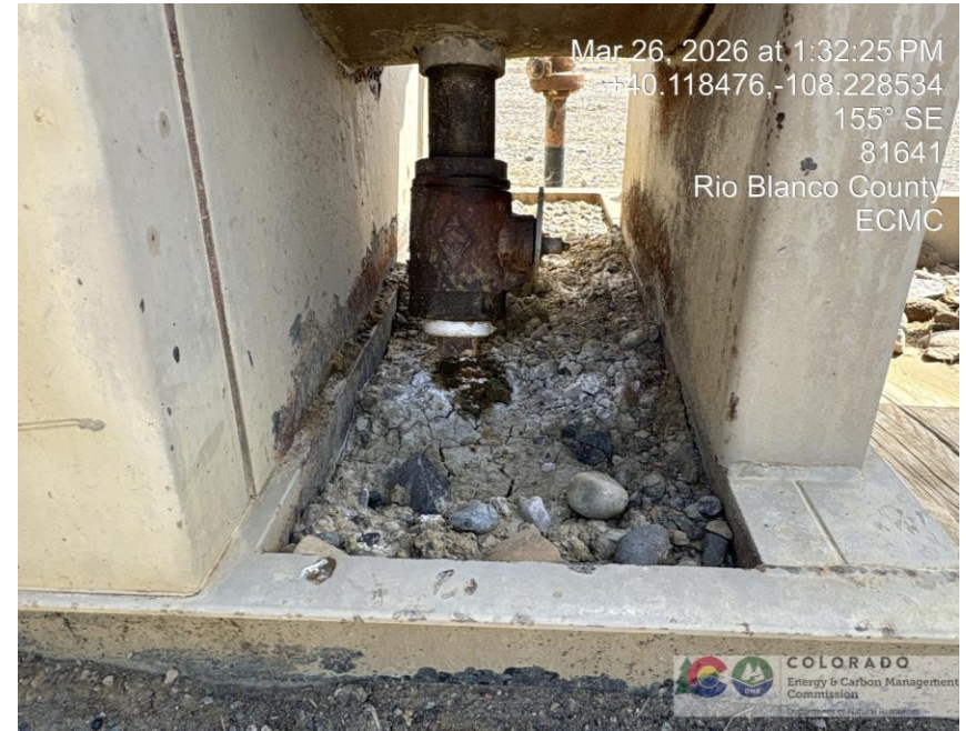
Photo # 3876 Stained soil beneath treater
