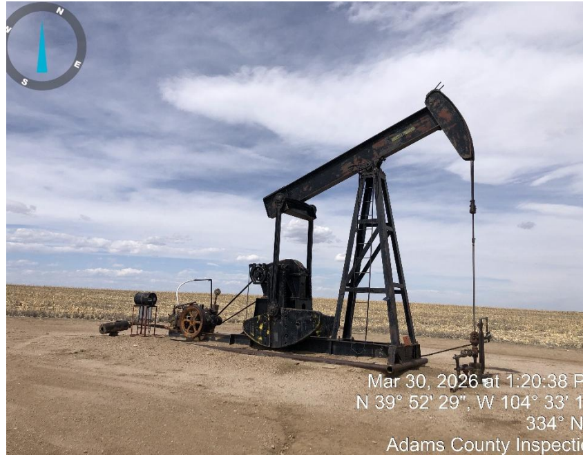
Photo #1 Pump jack.
