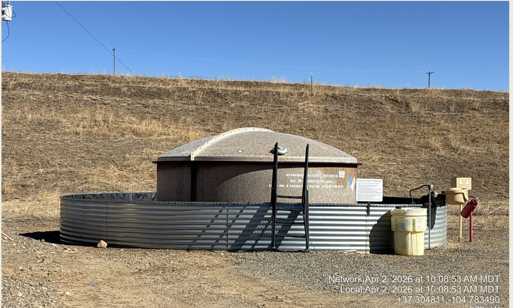
PHOTO 6: 210 BBL TANK BATTERY.
