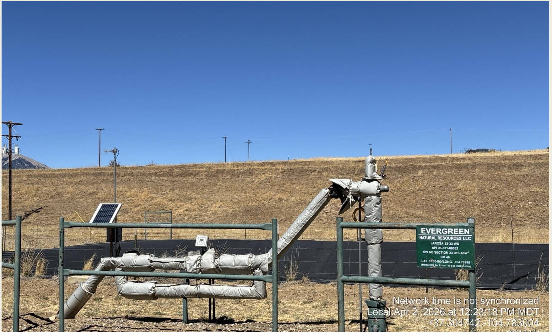
PHOTO 4: TR WELLHEAD AND EQUIPMENT.
