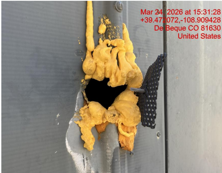
Wildlife Entry Hazard – Photo #03289
