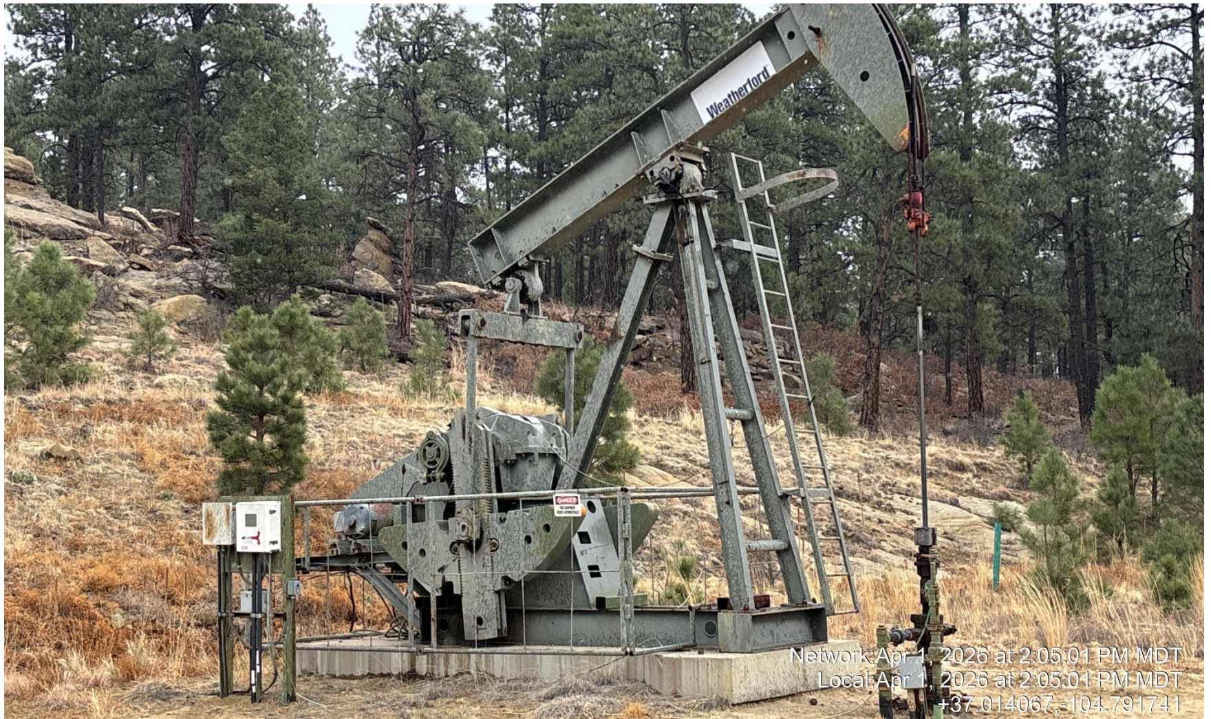
PHOTO 4: WELLHEAD AND EQUIPMENT.
