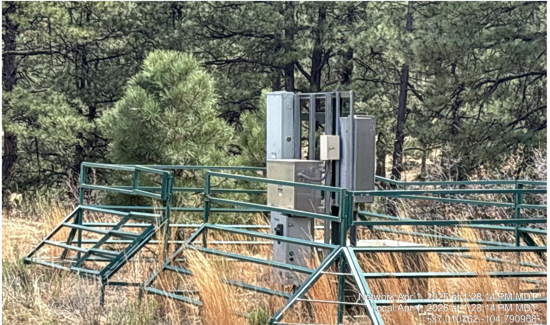
PHOTO 5: WEEDS NOT MAINTAINED INSIDE ELECTRIC PANEL FENCE. MAINTAIN WEEDS PER RULE 606. CA DATE 4/15/2026.
