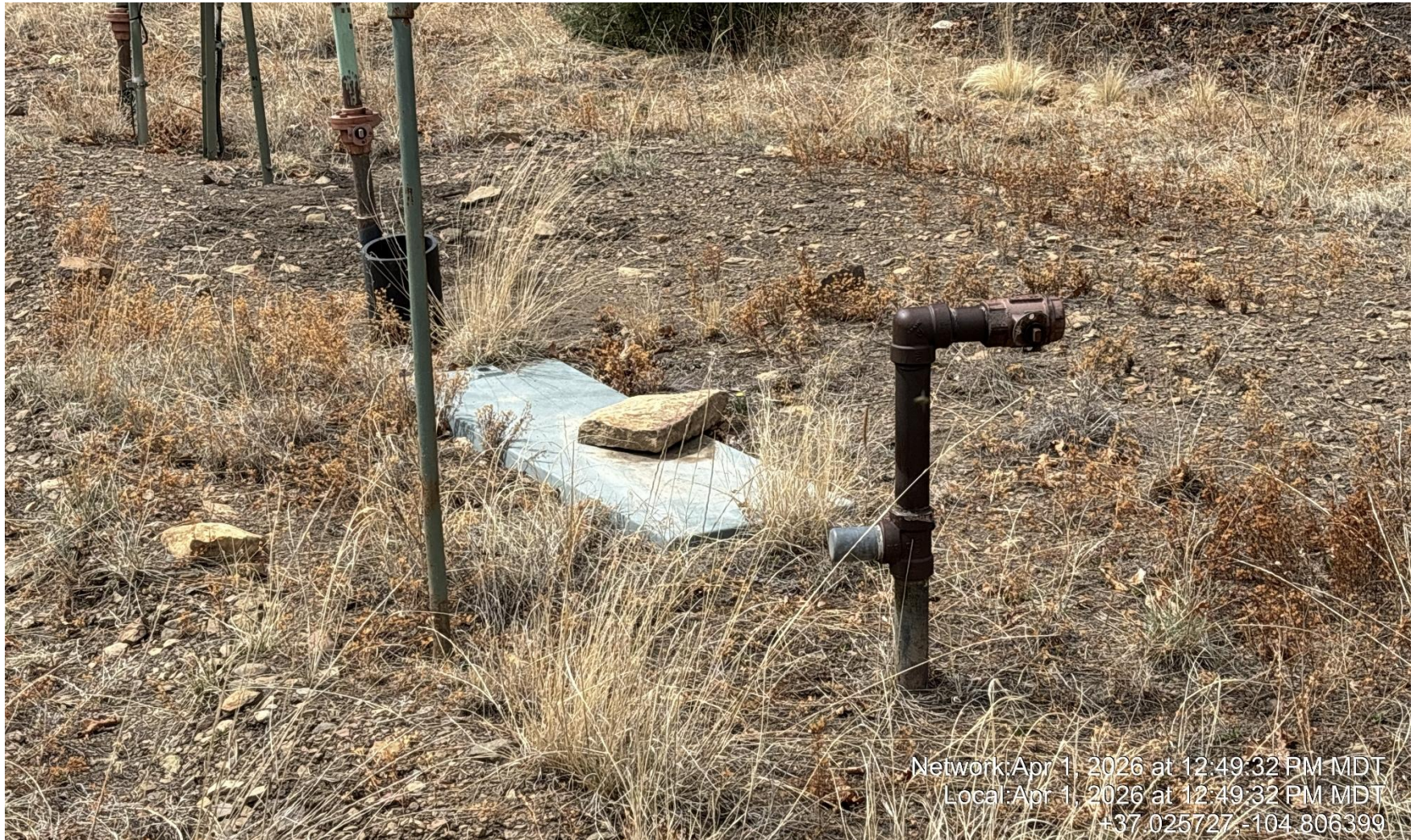
PHOTO 5: UNUSED EQUIPMENT ( 1-1" RISER AND 1-2" RISER NOT MARKED). REMOVE OR MARK RISER WITH CONTENTS (I.E. GAS, PRODUCED WATER) PER RULE 606. CA DATE 4/15/2026.
