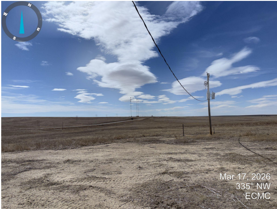
Photo 7. Electric service travels westbound along highway 36 from the well and tank battery location. It appears that the electric line served only this well and the former tank battery on the west side of county road U.
