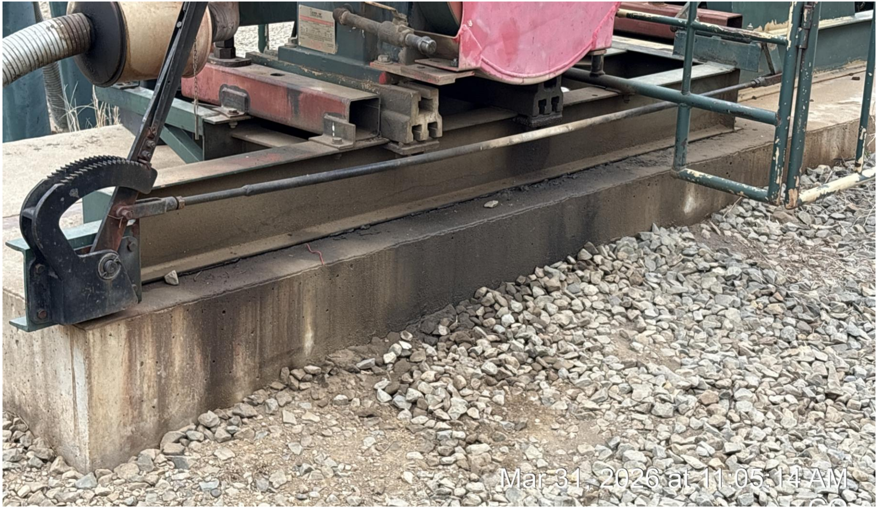
PHOTO 3: IMPACTED SOIL FROM MECHANICAL CONDITIONS
