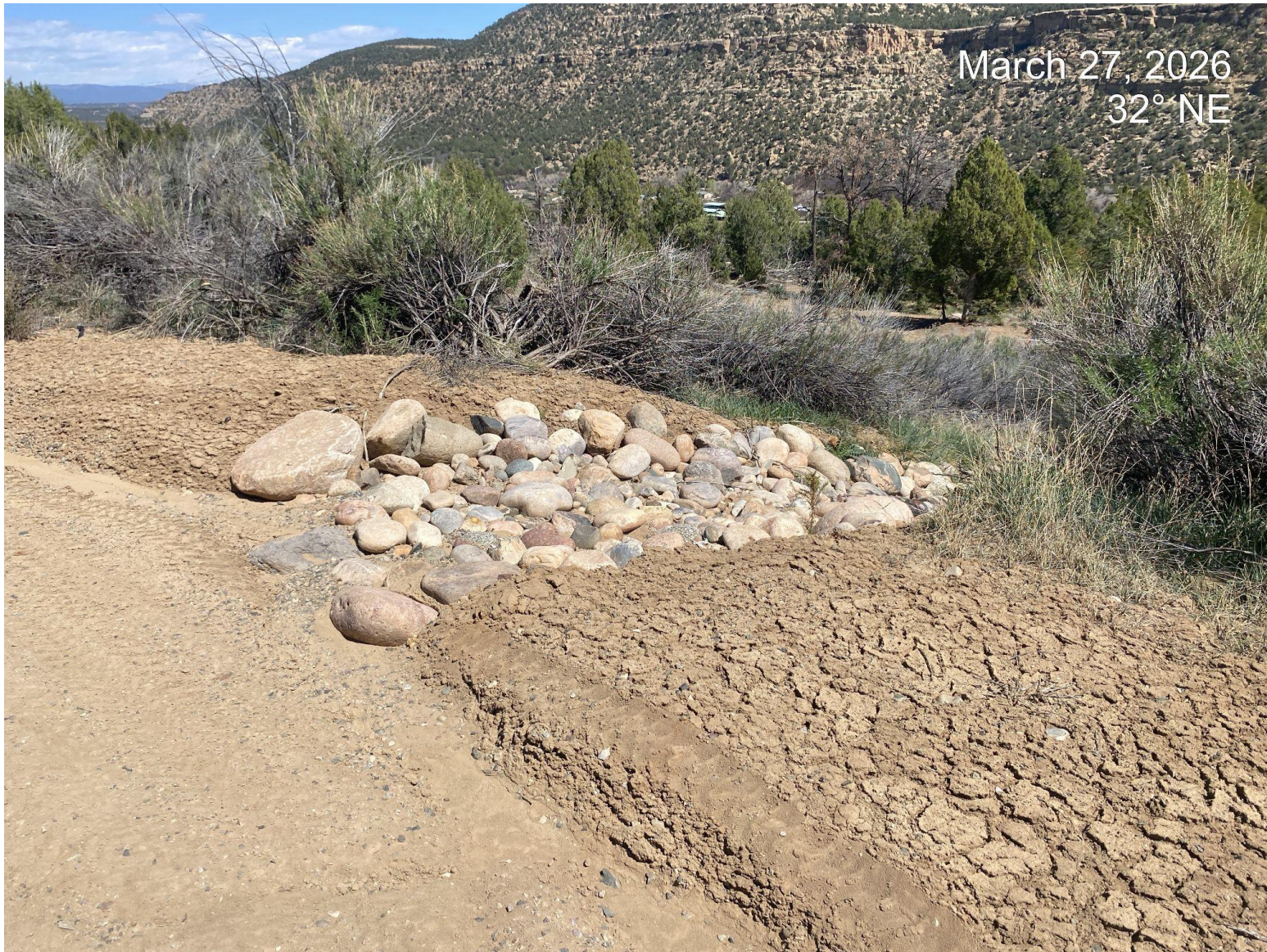
Photo 3. Stormwater BMPs installed on edge of active pad. No active erosion issues were observed during this inspection.
