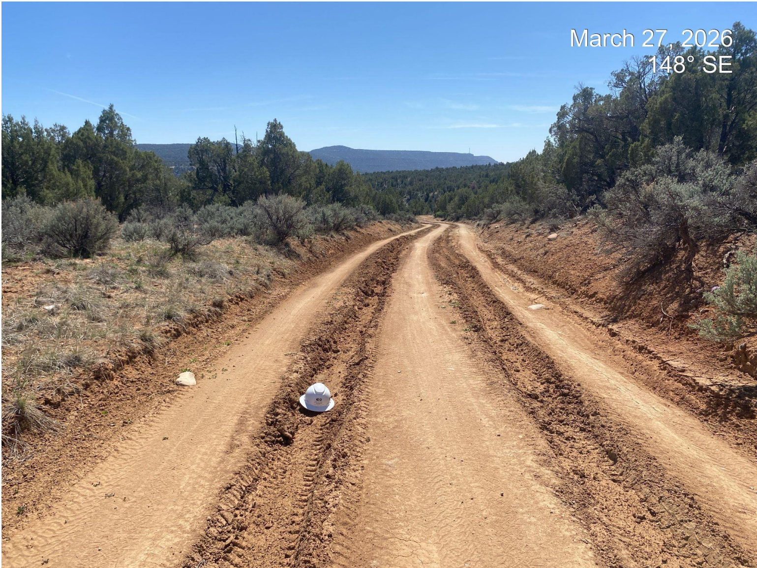
Photo 3. View of deep rutting occurring on the access road.
