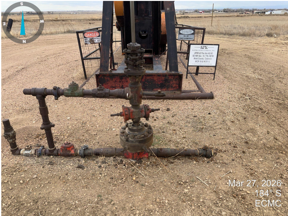
Photo 1. Photo taken at the wellhead looking south.
