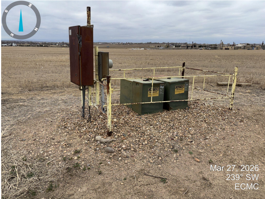
Photo 3. Electric equipment on location.
