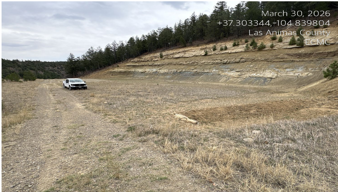
Photo 4. Facing southeast at the location. The location has not been recontoured and a steep cut slope remains. Previous corrective action not completed.
