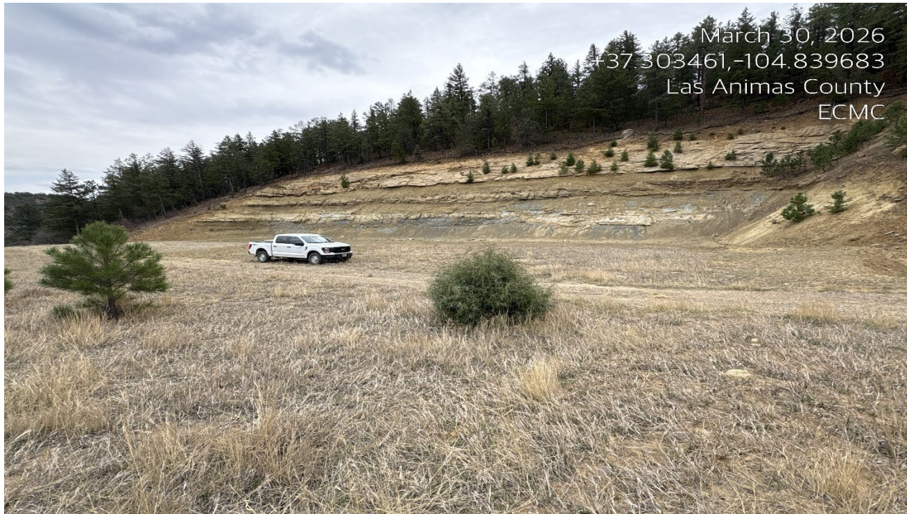
Photo 2. Facing southeast at the location. The location has not been recontoured and a steep cut slope remains. Previous corrective action not completed.
