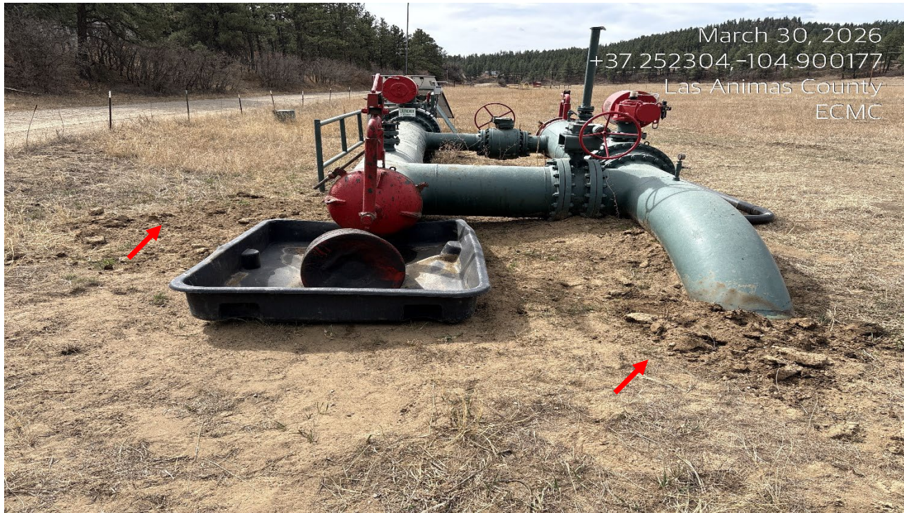
Photo 2. There is impacted material shown at red arrows that needs to be cleaned up.
