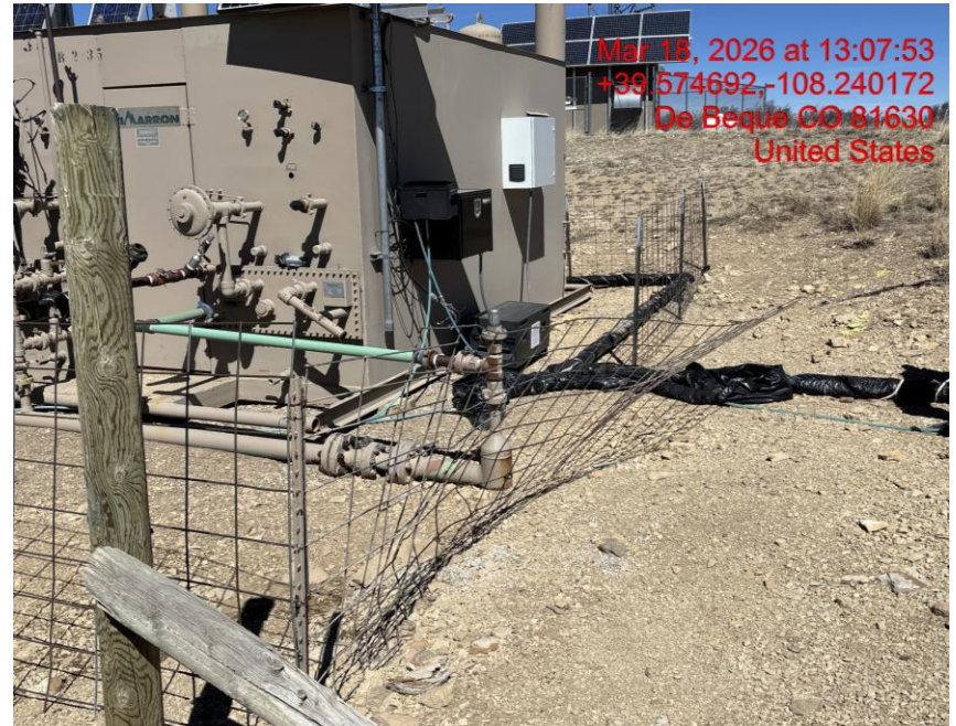
Damaged Fencing – Photo #03216
