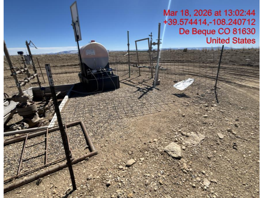
Damaged Fencing – Photo #03196
