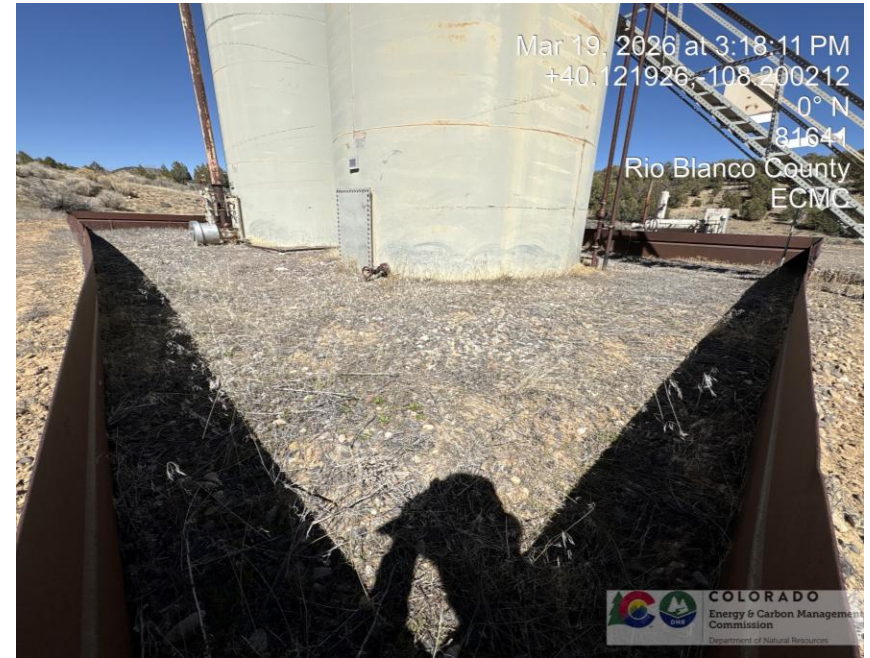
Photo # 3471 Dead weeds/debris
