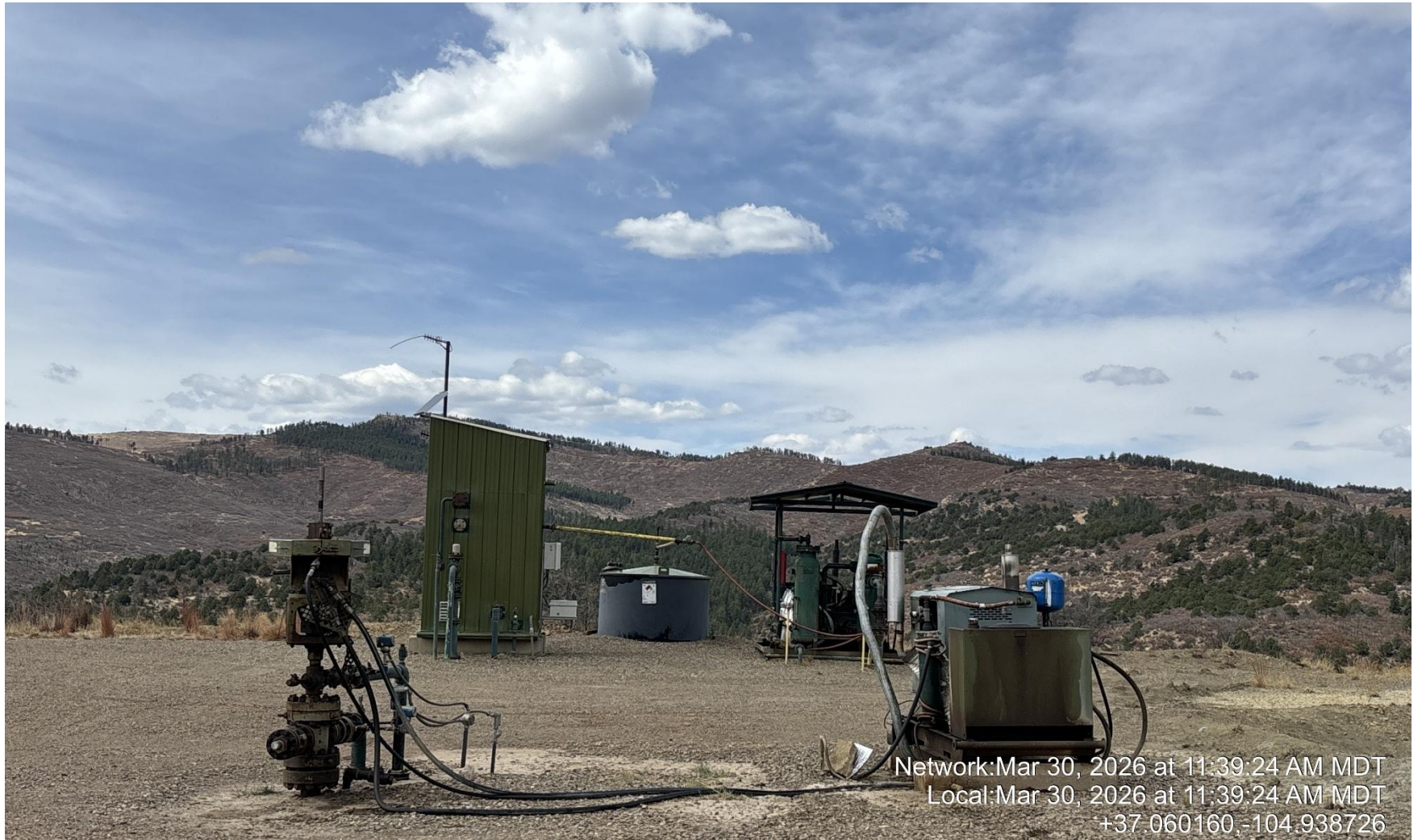
PHOTO 4: WELLHEAD AND EQUIPMENT.
