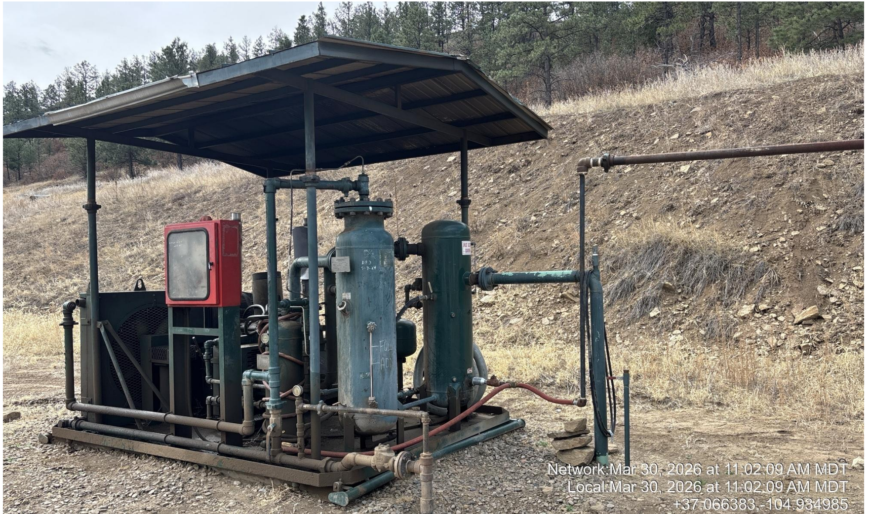
PHOTO 5: Vacuum pump observed on well without ECMC approval. Provide ECMC with documentation showing approval of use of vacuum pump. CA DATE 4/15/2026.
