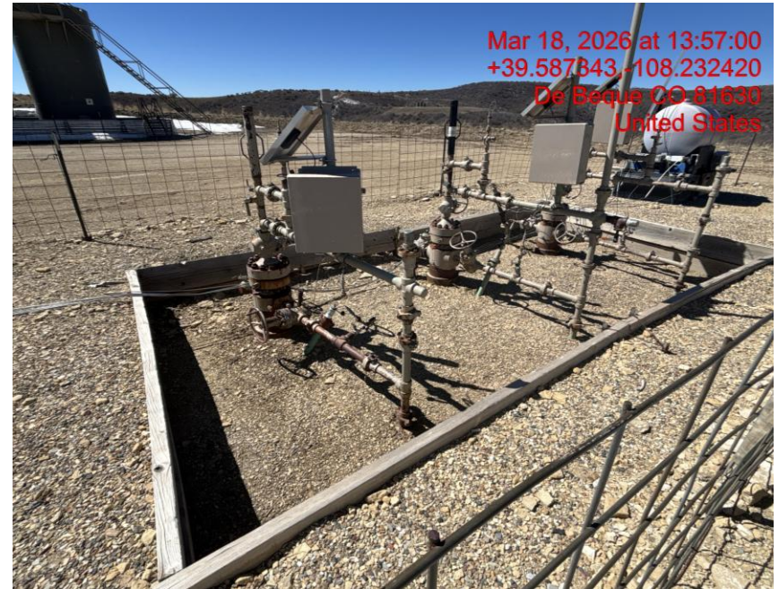
No Wildlife Egress in Wellhead Cellar – Photo #03259
