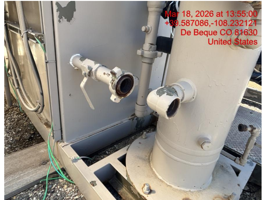
Open-Ended Lines/Wildlife Entry Hazard – Photo #03254
