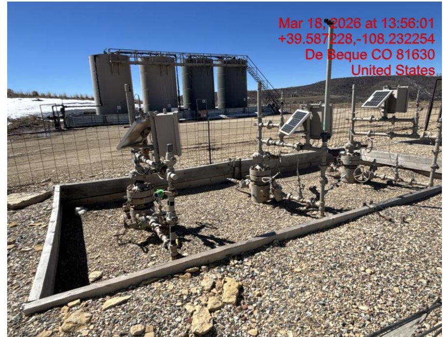
No Wildlife Egress in Wellhead Cellar – Photo #03257
