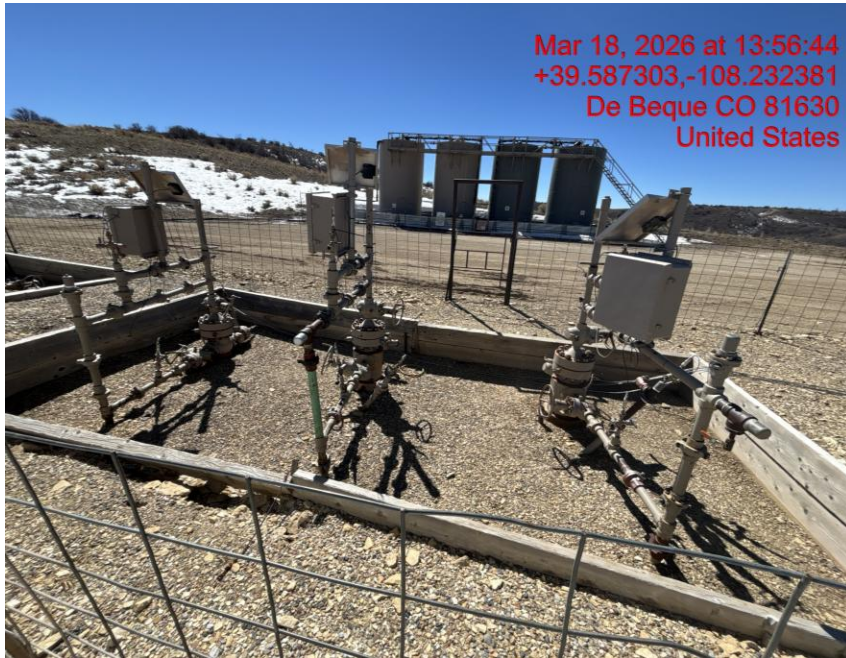
No Wildlife Egress in Wellhead Cellar – Photo #03258
