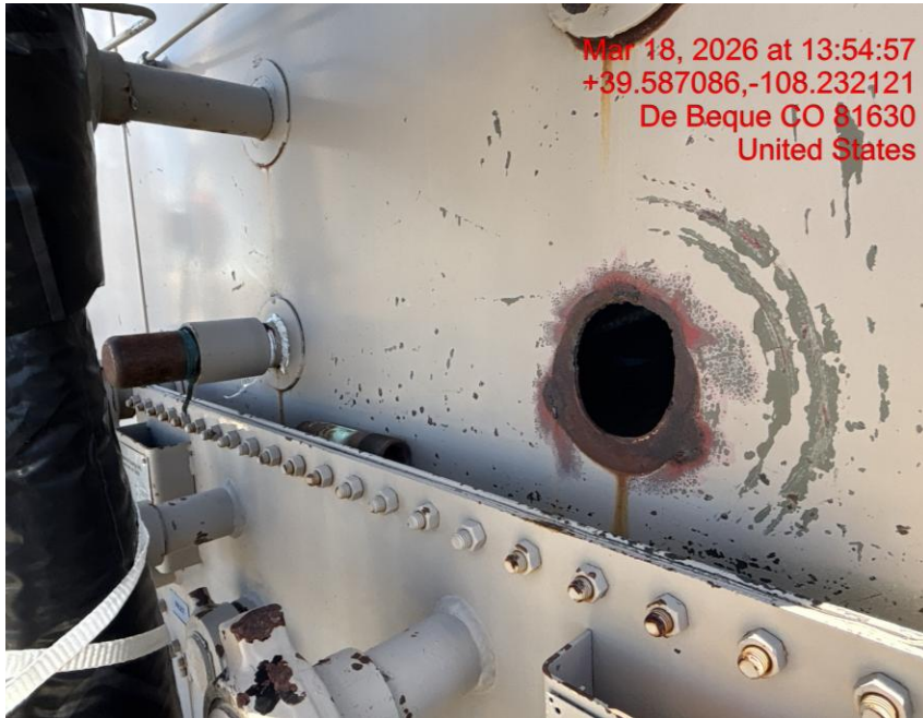
Wildlife Entry Hazard – Photo #03253
