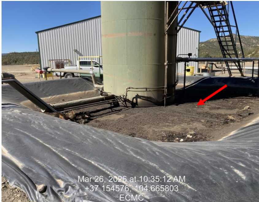
Photo 18: TB # 1 Lower Level, oily residue in containment
