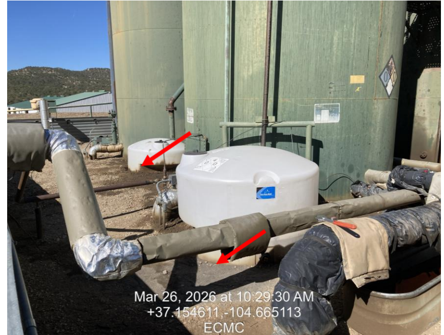
Photo 13: TB # 1 on middle level, oil-stained soils
