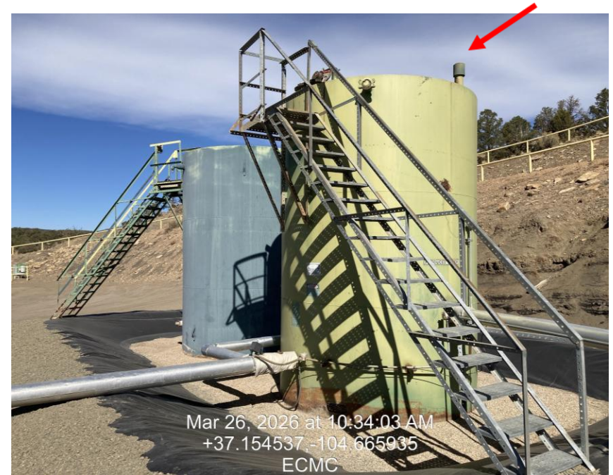
Photo 19: TB # 2 Lower Level, Missing Bird Protector
