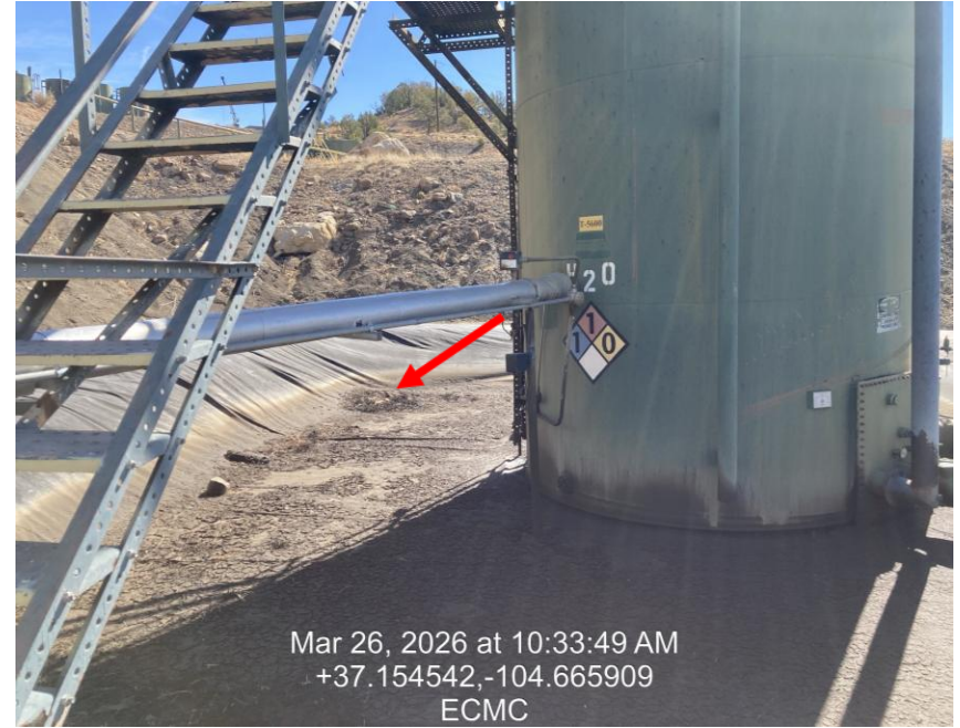
Photo 17: TB # 1 Lower Level, oily residue in containment
