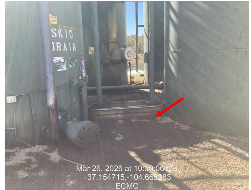
Photo 15: TB # 1 on middle level oil-stained soils
