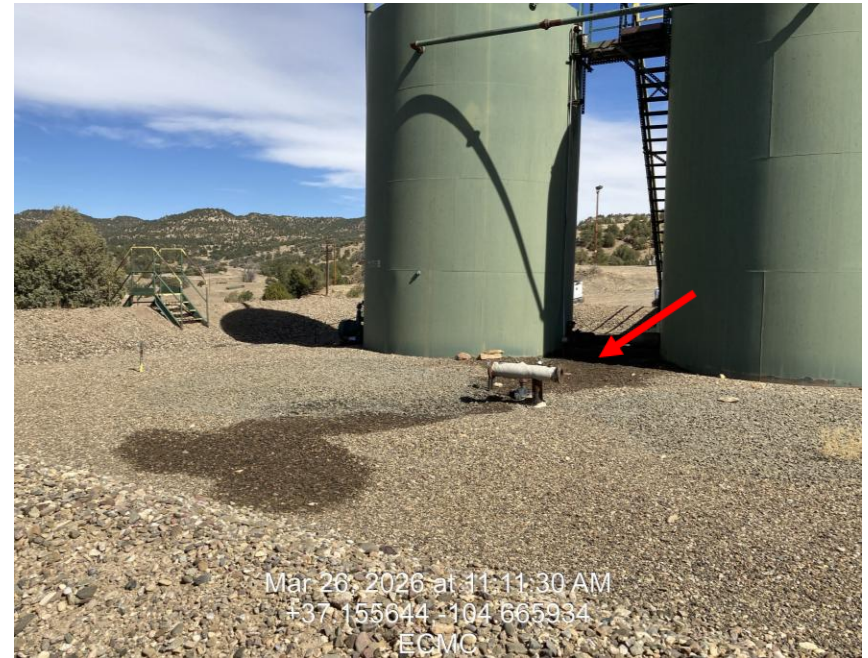
Photo 21: TB within compressor footprint, oil-stained soils.
