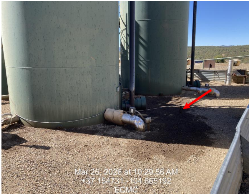
Photo 14: TB # 1 on middle level oil-stained soils
