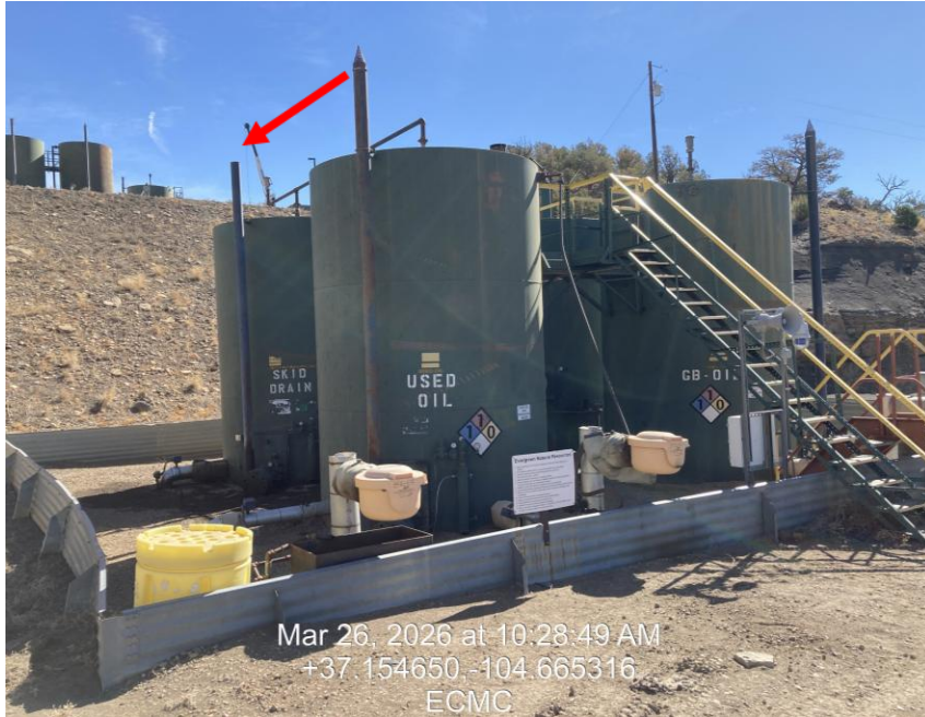
Photo 13: TB # 1 on middle level, missing bird protector
