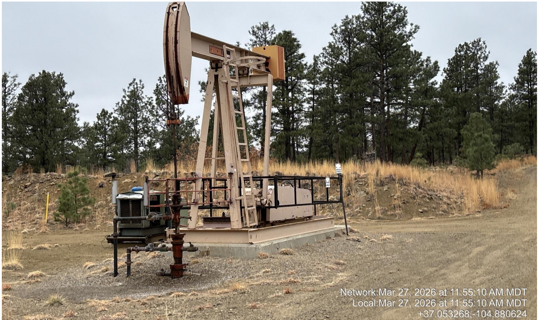
PHOTO 5: V WELLHEAD AND EQUIPMENT.
