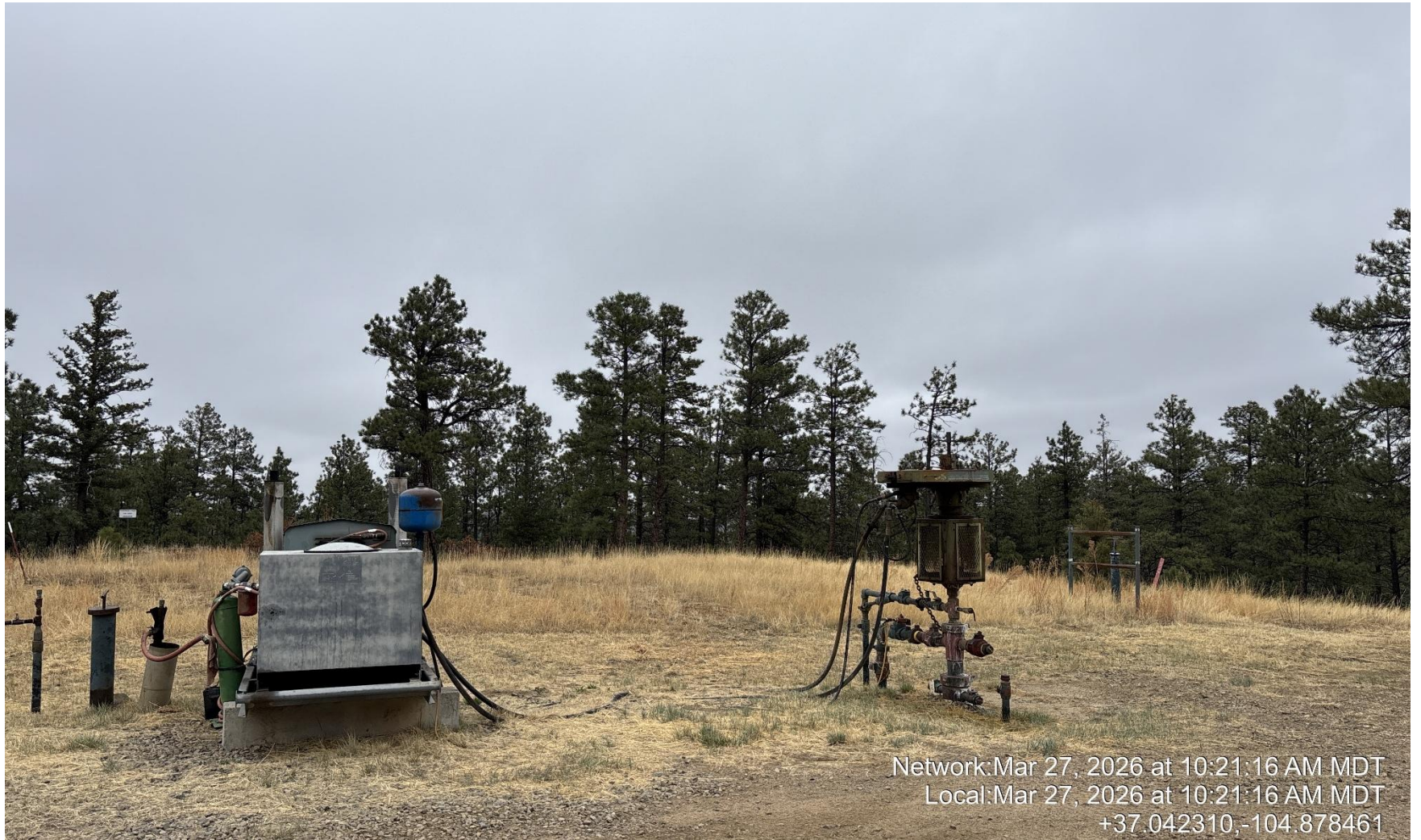
PHOTO 4: R WELLHEAD AND EQUIPMENT.
