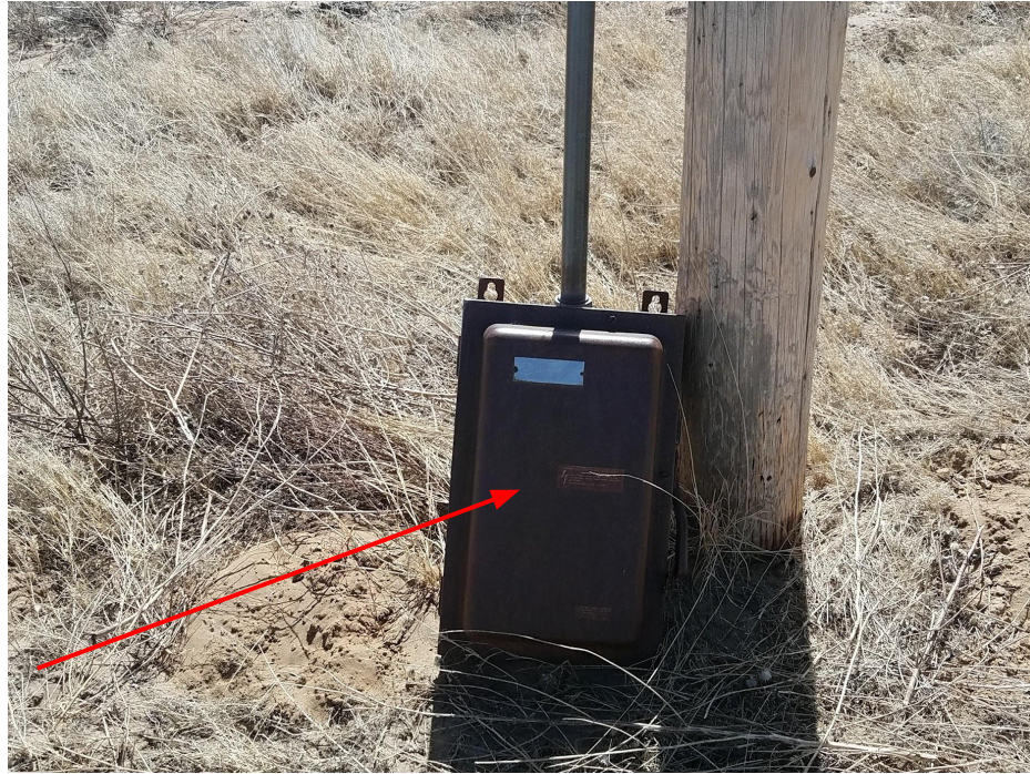
Photo 5. Photo taken from the well location, illustrating unused utility equipment.
