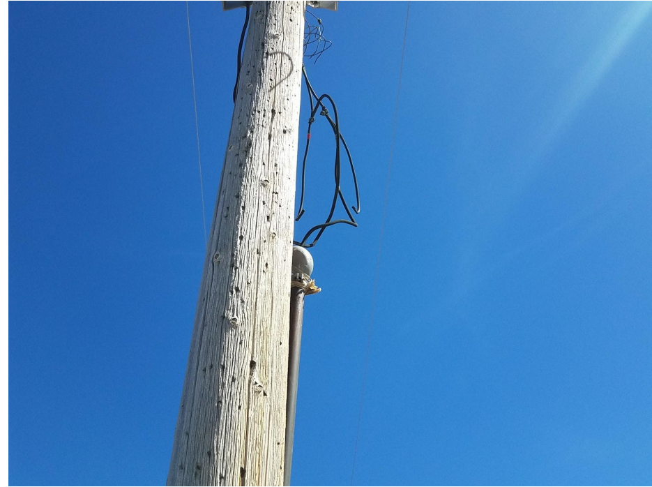
Photo 6. Photo taken from the well location. Photo illustrates the utility power has been disconnected and is no longer in use.
