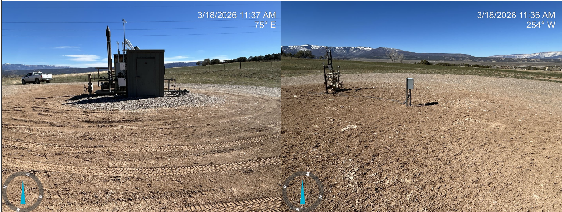
Photo 2: Photos showing an overview of the location looking east and west, respectively.
