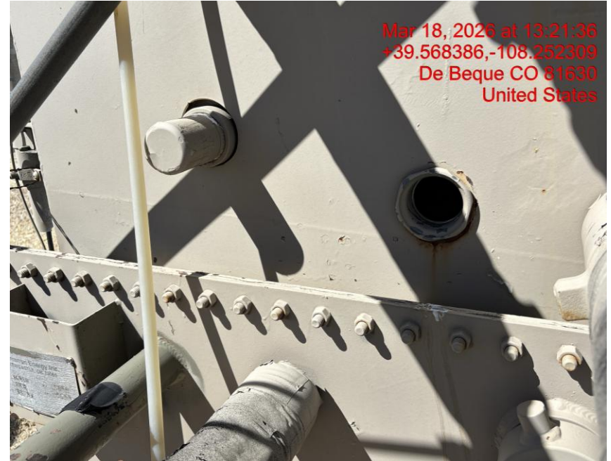
Wildlife Entry Hazard – Photo #03225
