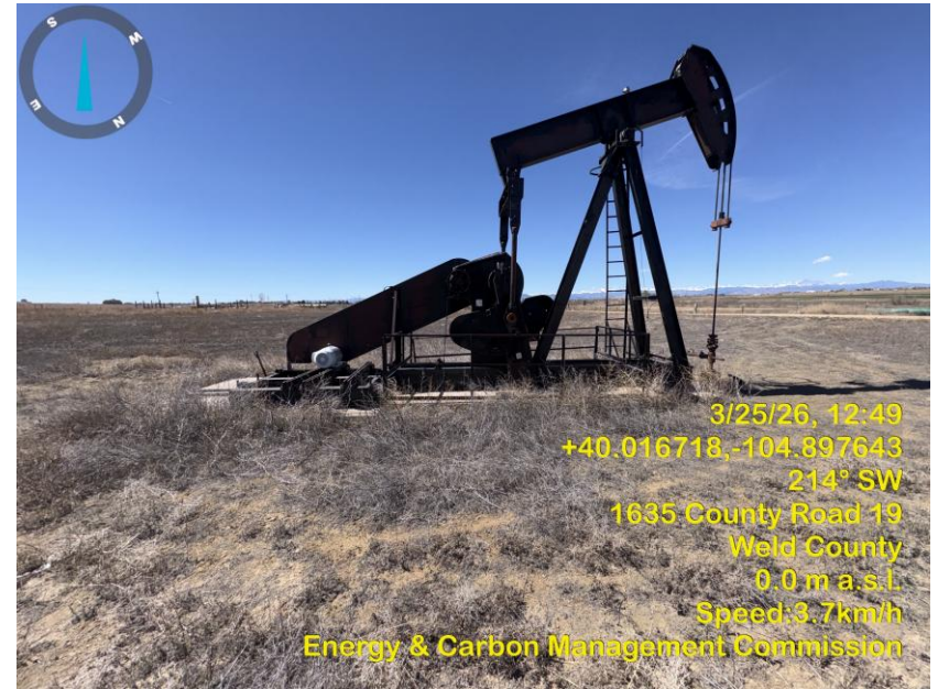
Photo 4 Wellsite pump jack.
