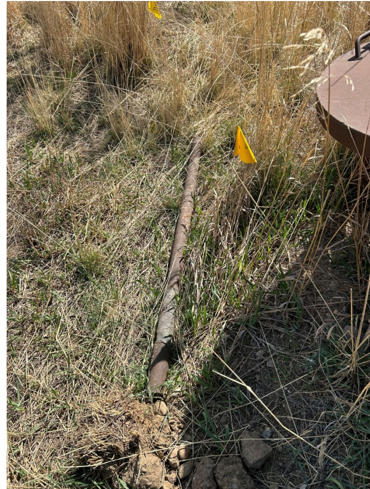
Photo 6: Unused pipe debris east of southern valve can.
